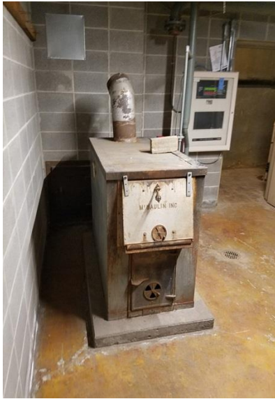
Abandoned Mechanical Equipment
