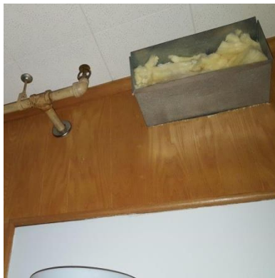
Exposed Pipes and Abandoned Duct at Storage Room
