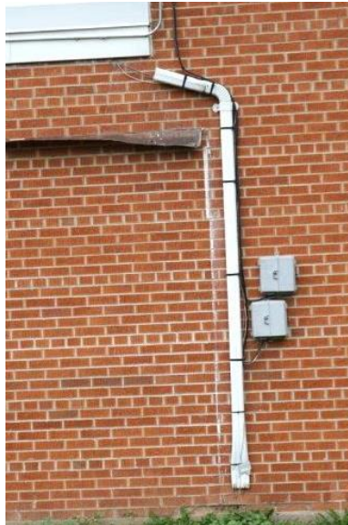
Gutter Assembly Used as Conduit, Exposed Wires
