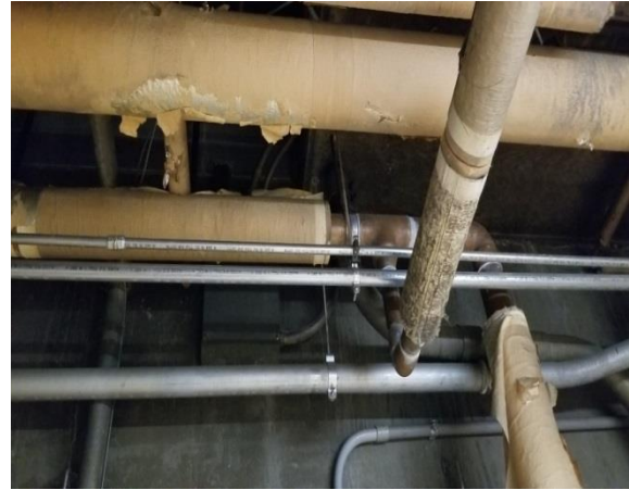
Plumbing Piping with Asbestos
