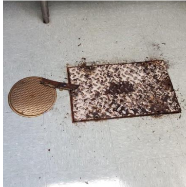
Rusted Kitchen Metal Floor Plate
