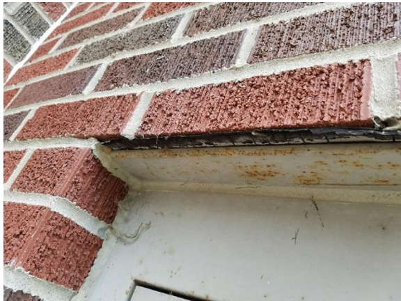
Rusted Lintel, Deteriorated Caulk/Flashing
