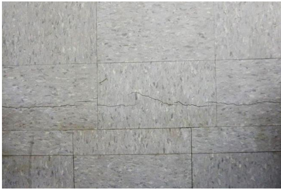
Cracked Vinyl Tile at Art Room
