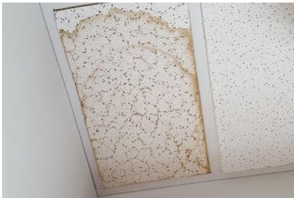
Ceiling Tile Stained at Corridor
