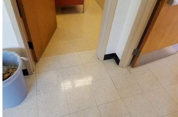
Vinyl Tile Delamination; No Transition
