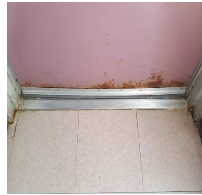
Rust Forming at Base of Exterior Door
