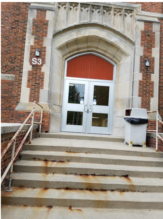
Exposed/Rusted Steel at Stair Risers
