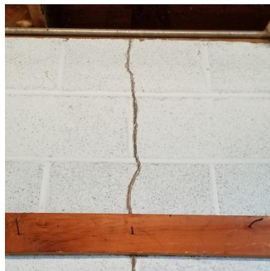
Cracking CMU Wall at Storage Room
