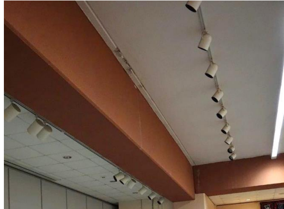
Ceiling/Bulkhead Staining From Leaking Roof
