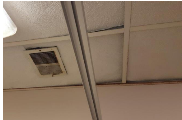
Ceiling Tile Rusted & Damaged at Men's Restroom
