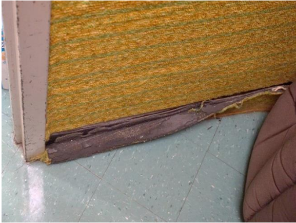
Damaged Fabric Wall Covering/Base
