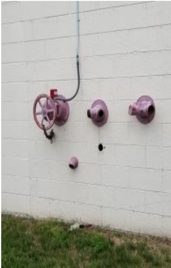
Stand Pipe/Valve for Sprinkler System
