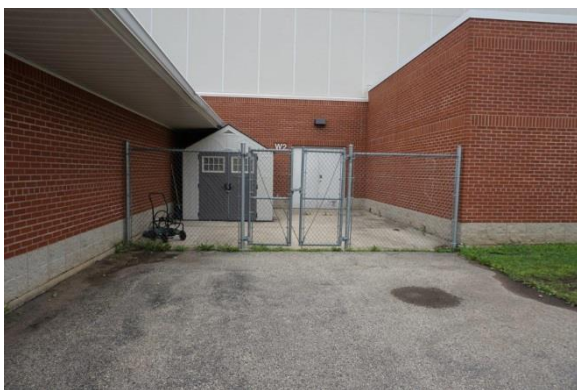
Egress Route Blocked at Exit W2
