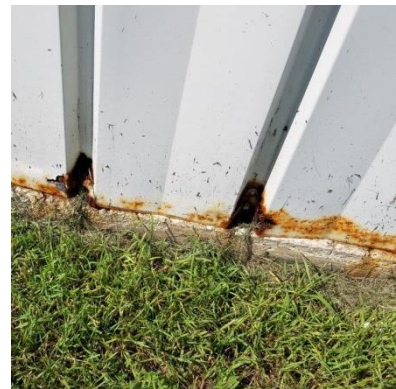
Rusted Metal Siding at Base
