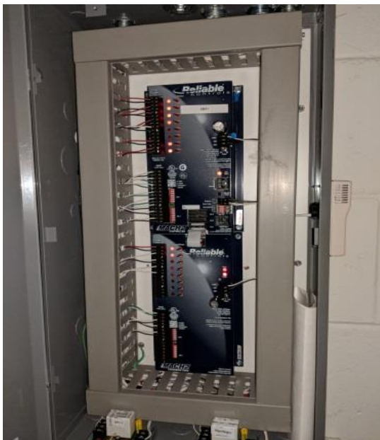
Reliable Controls Main Panel
