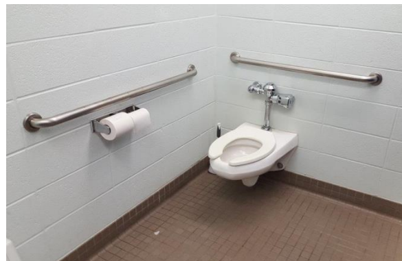
Missing Vertical Bar at Women's Restroom
