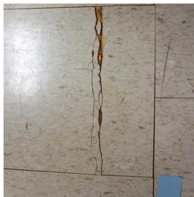
Cracked/Deteriorated Vinyl Tile
