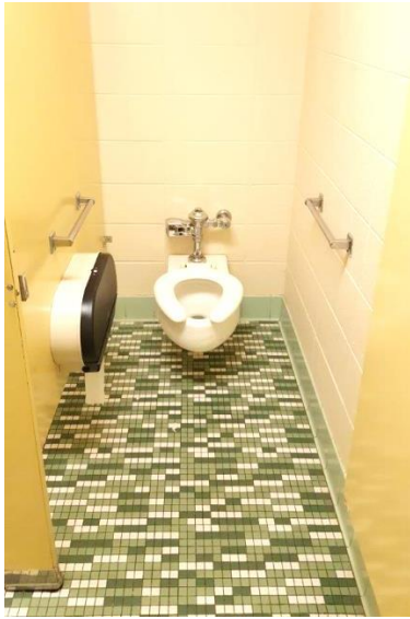
Missing Grab Bars; Non-ADA Compliant Clearances
