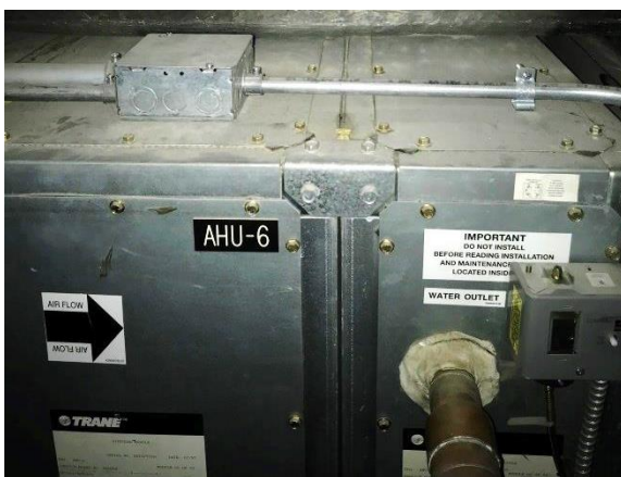
Air Handling Unit 6 - Serves Gymnasium
