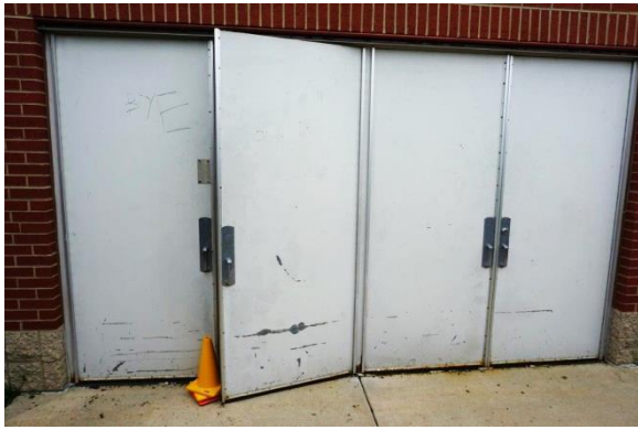
Scratches/Dents on Exterior Doors
