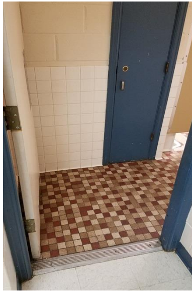
Non-ADA Compliant Entry at Girl's Restroom
