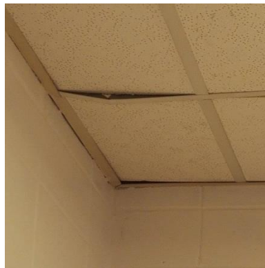
Ceiling Tile Sagging at Music Room
