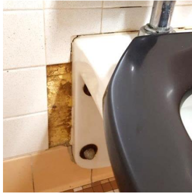
Missing Tiles Around Toilet Fixture
