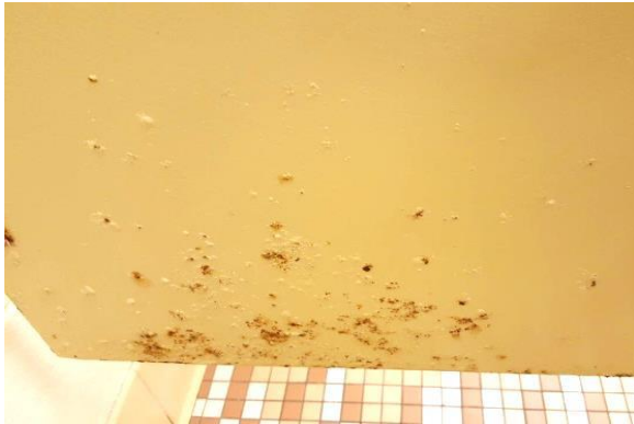
Rusting Toilet Partition
