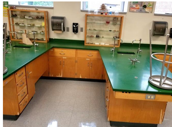
Damaged Base Cabinets at Room 306
