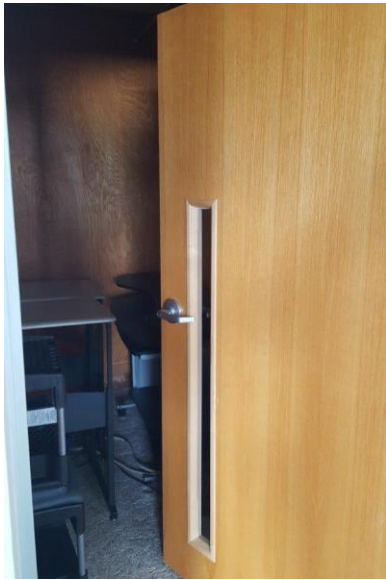
Door Installed Upside Down at Storage Room
