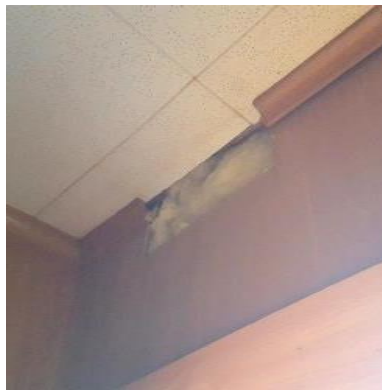
Exposed Insulation at Storage Room
