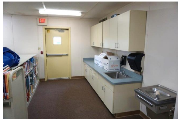
Non ADA Compliant Casework at Room 113
