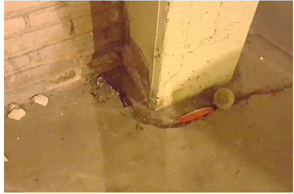
Large Crack at Column Floor Base at Boiler Room
