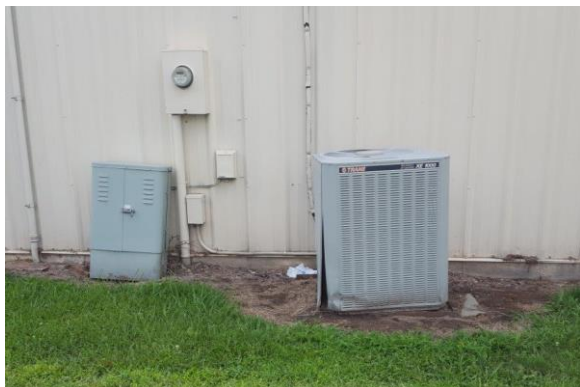
Displaced Electrical & Mechanical Units
