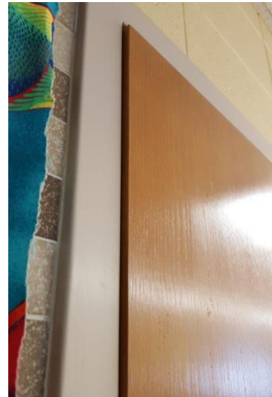
Door Doesn't Close Properly at Kindergarten 112 Bathroom
