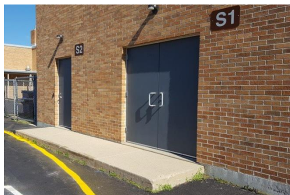
W-1 Not ADA Compliant - Missing ramp and handrails
