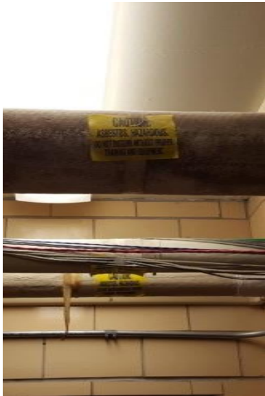
Asbestos on Mechanical Pipes
