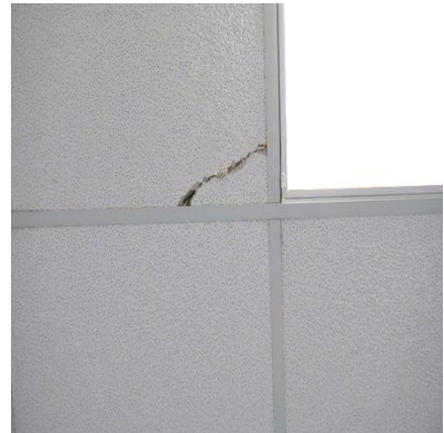
Damaged Ceiling Tile
