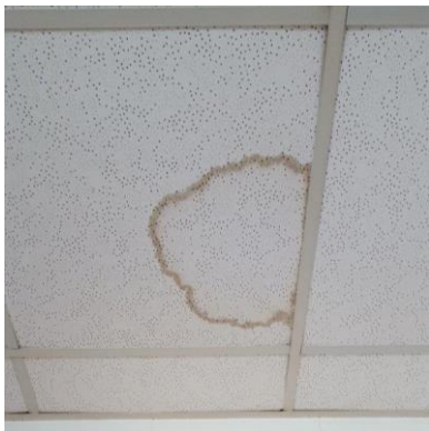
Ceiling Tile Staining at Kindergarten Room 100
