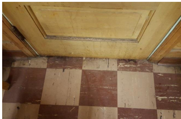
Non-ADA Compliant Door Width at Toilet Room; Possible Asbestos in Vinyl Tile
