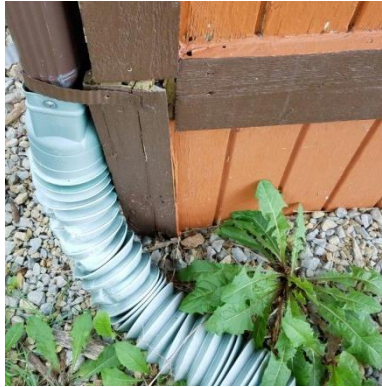
Wood Trim Deteriorating at Base
