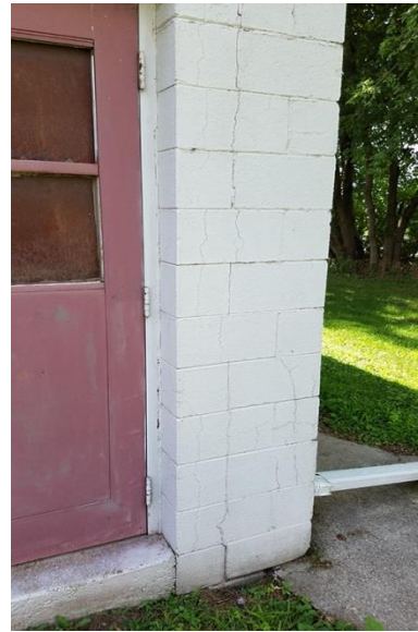
Cracking at CMU Corner
