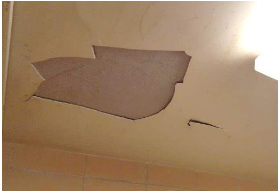
Deteriorated Plaster Ceiling at Restroom
