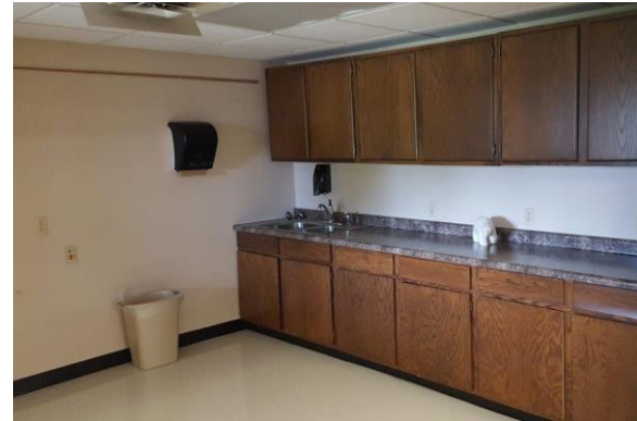
Non-ADA Compliant Counters/Fixtures at Conference Room
