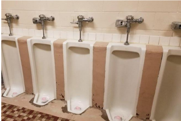
Flaking Paint at Boys Restroom Floor
