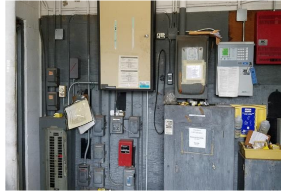
Electrical Panel Mounting Location
