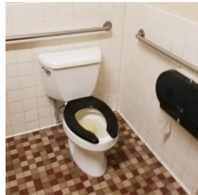
Missing Vertical ADA Grab Bar at Girls Restroom
