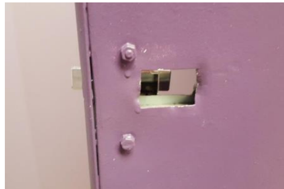
Missing Stall Lock at Women Restroom 109
