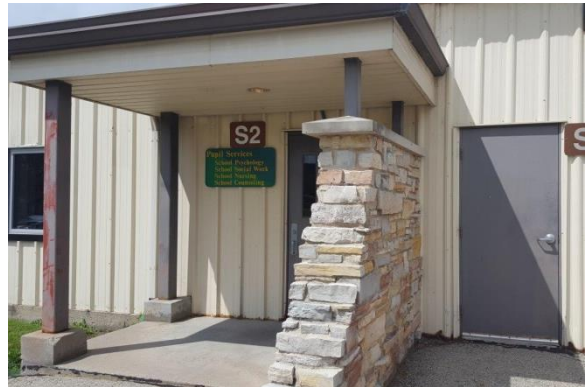
Non-ADA Compliant Entry at District Instructional Media Center Entrance
