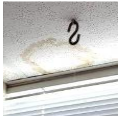
Ceiling Tile & Grid Degradation at Grade 2 - Room 100
