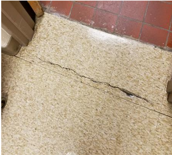
Damaged Vinyl Tile at Room Entry
