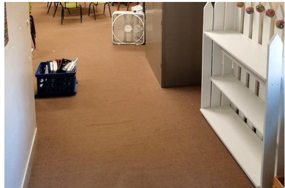
Carpet Stained and Delaminating at Classroom 204
