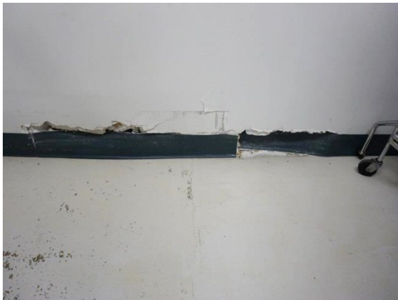
Damaged Wall and Base
