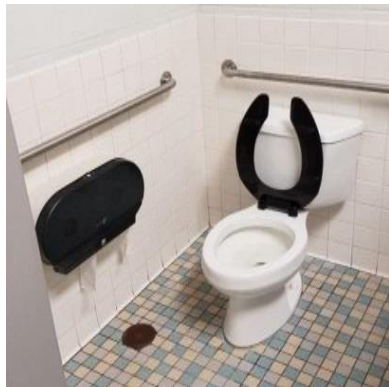
Missing Vertical ADA Grab Bar at Boys Restroom
