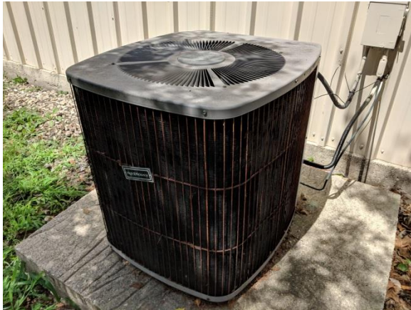
Carrier Air Cooled Condensing Unit
