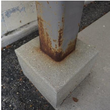
Rusted Column Post
