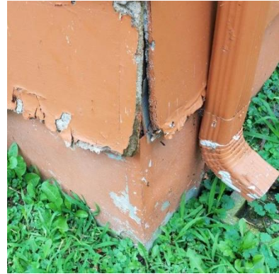
Wood Siding Deteriorating At Base
