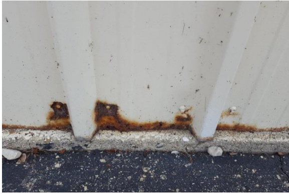
Rusted & Dented Siding
