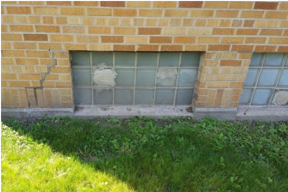
Damaged & Patched Glass Block Windows; Masonry Repairs
