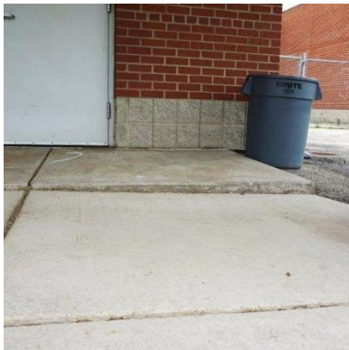
Heaving Concrete Walks
