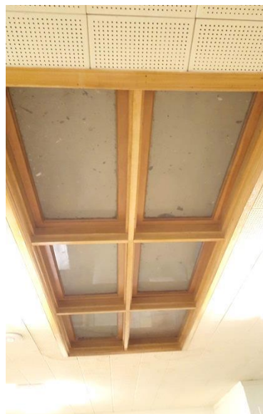
Abandoned Sky Light at Toilet Rooms
