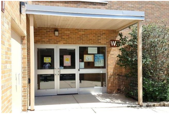
Resting at Base of Columns at W-2 Entrance; Heaving Concrete Walk
