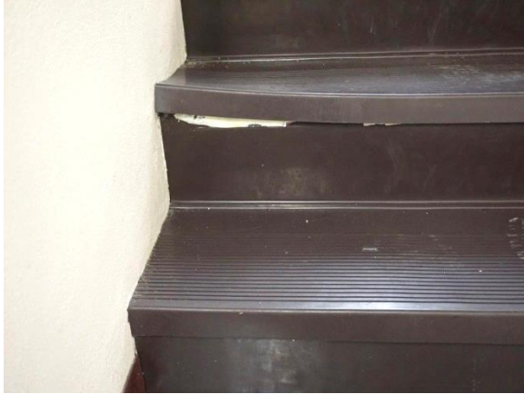
Delaminating Stair Tread
