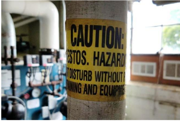
Asbestos Notification on Piping
