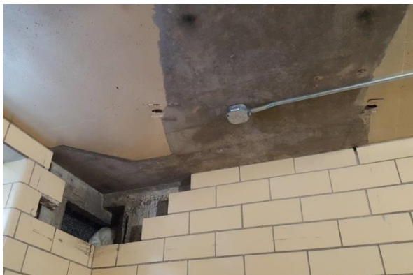
Ceiling/Wall Damage for created Mechanical Opening
