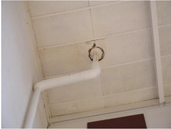
Roof Leak at Roof Drain/Conductor
