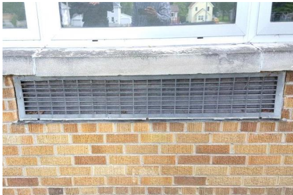
Rusted and Damaged Exterior Unit Vent Louver
