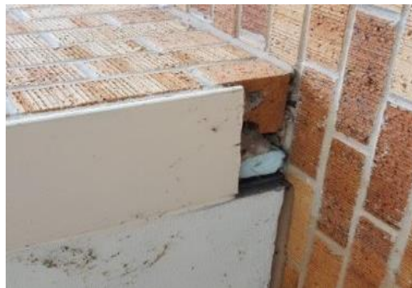
Exposed Cavity Wall/Deficient Lintel
