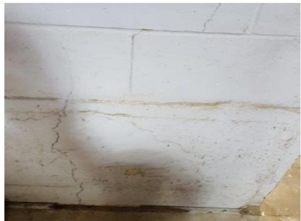
Cracks on Exterior CMU Wall
