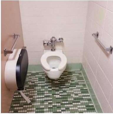
Incorrect/Missing Grab Bar Locations at Girl's Restroom; Clearance Issues
