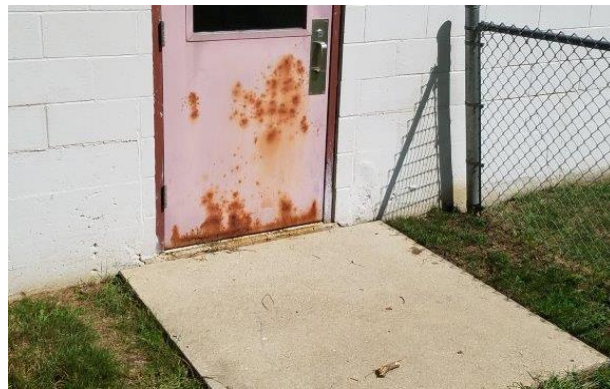
Rusted Exterior Door
