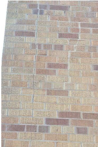
Cracking along Masonry Wall
