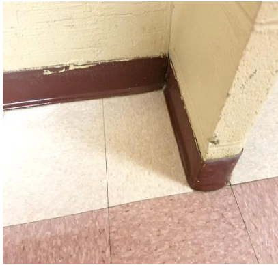
Base Delamination and Damage
