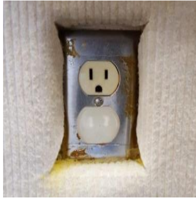
Outlet Enclosed by Padding & Visible Corrosion at Classroom 116
