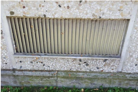
Deteriorated Louver at Unit Vent at S-3 Entrance
