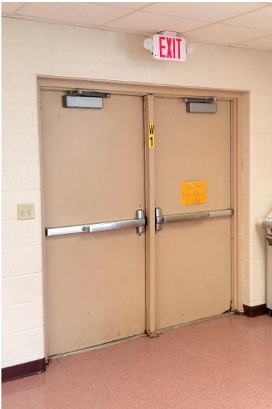
Rusting Exit Door at Multipurpose Room
