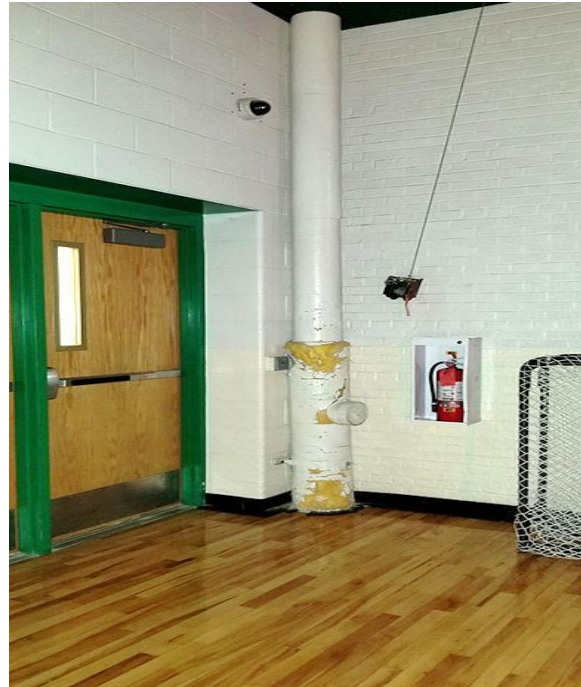
Missing/Damaged Insulation at Roof Conductor
