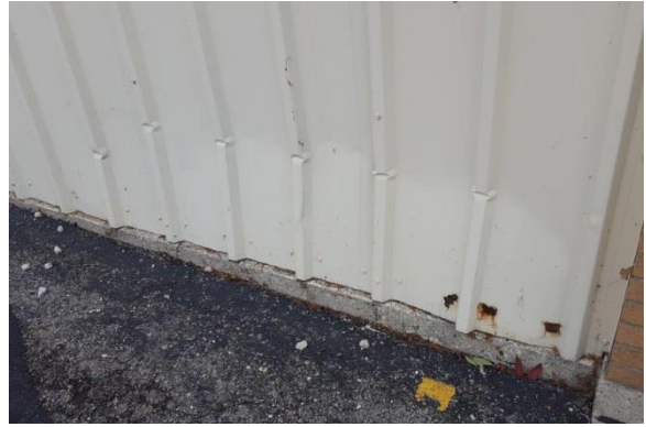
Rust at Base of Siding Walls
