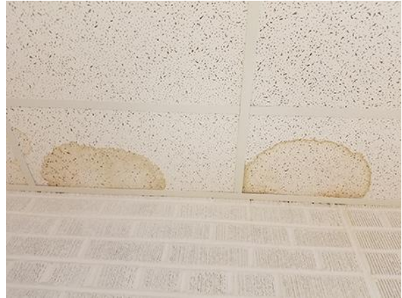
Ceiling Tile Staining at Library
