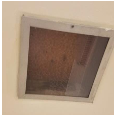
Abandoned Sky Light Boys Restroom
