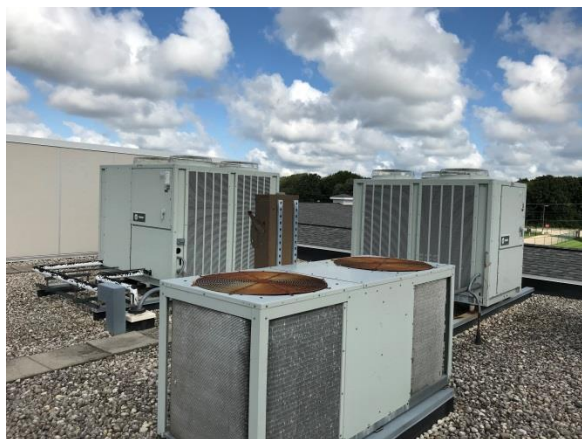
Air Cooled Condensing Units on Roof
