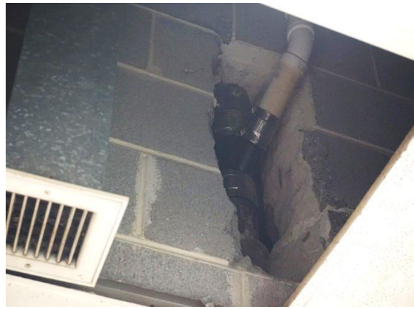
Missing Ceiling Tile Exposing Plumbing Penetration into Masonry Wall
