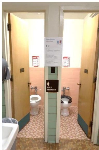
Door Width Doesn't Meet ADA Standards at Staff Lounge 227
