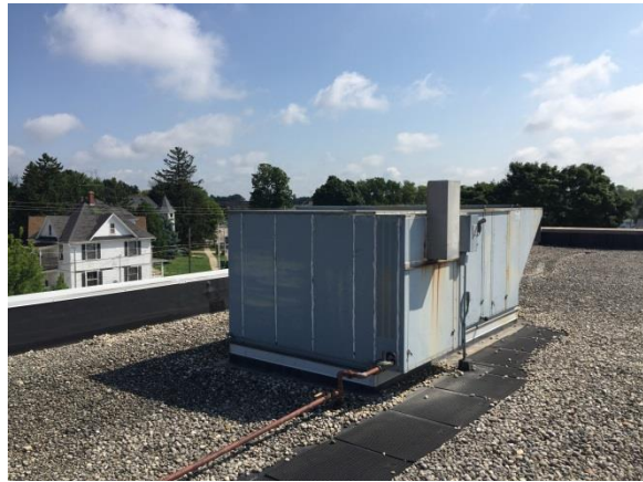
Engineered Air Make-up Air Unit
