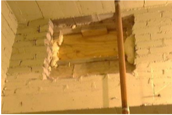
Loose Masonry at Opening at Boiler Room
