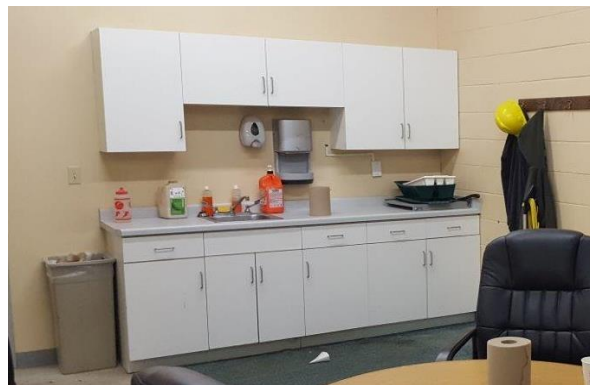
Non-ADA Compliant Casework/Sink at Break Room
