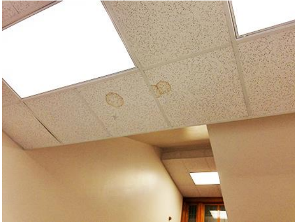
Ceiling Tile Staining at Stair S3
