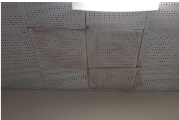
Ceiling Tile Staining, Sagging, and Deteriorating at Classroom 207
