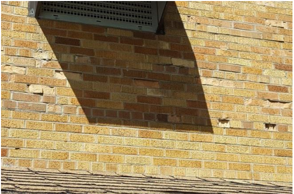
Spalling Brick Above Roof Area
