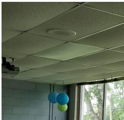
Ceiling Tile Sagging at Classroom 100
