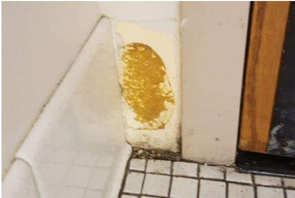
Missing Tile Base at Girls Restroom
