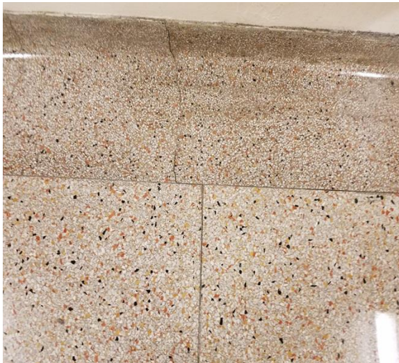
Cracked Terrazzo at Corridor
