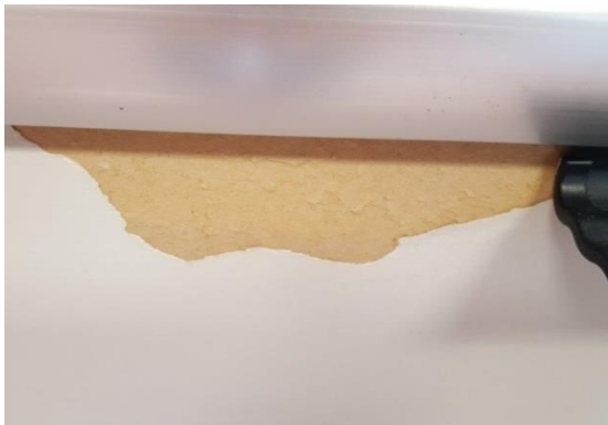
Damaged Gypsum Wall at Classroom
