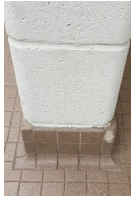
Tile Base Damaged
