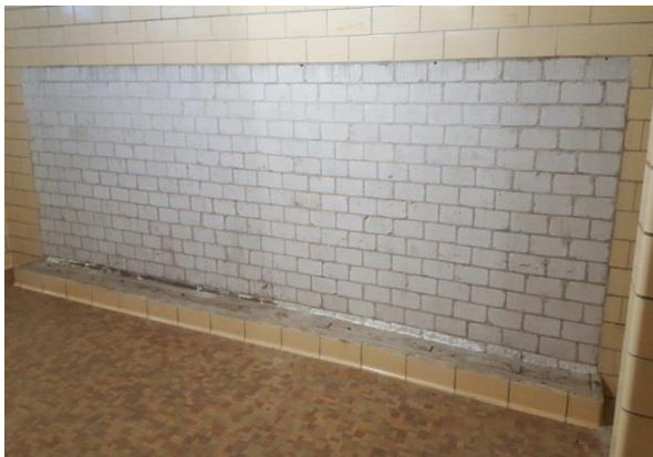
Cracks on CMU Wall at Removed Lockers at Locker Rooms
