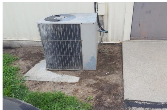
Displaced Mechanical Unit
