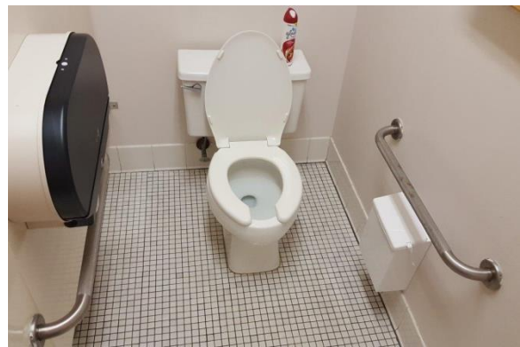
Missing Vertical Bar and Clearance Issue at Men's Restroom
