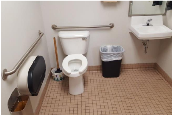
Missing Vertical Grab Bar at Faculty Restroom
