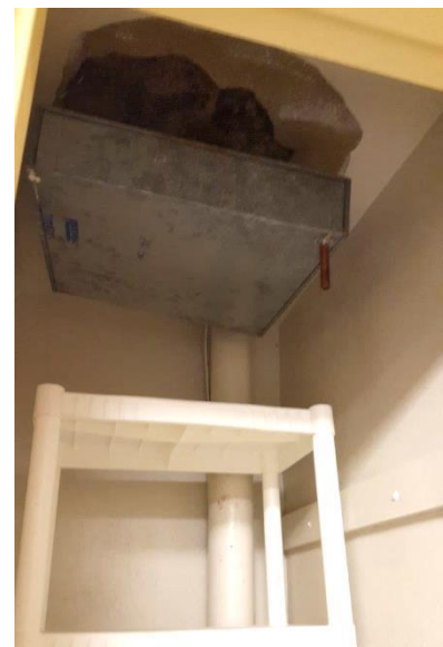
Fabricated Water Collector at Staff Lounge 227
