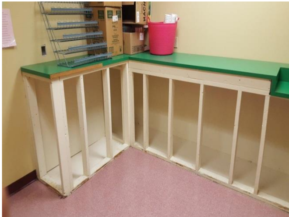
Damaged PLam Counter/Base
