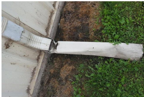
Damaged & Dented Downspout & Extension
