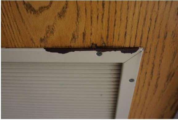
Rust on Door Louver at Men Restroom
