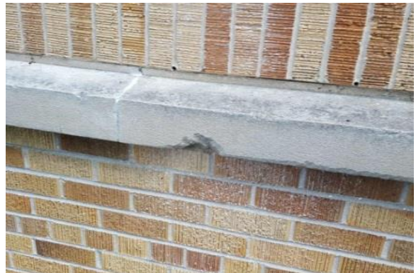
No Weeps Installed at Concrete Sill
