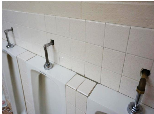
Missing Escutcheon around Plumbing Pipes
