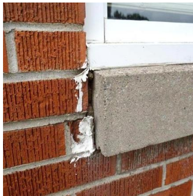
Improper Flashing Installation at Window Sill
