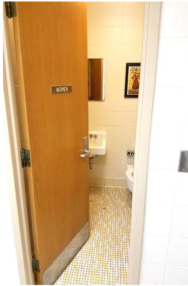
Non-ADA Compliant Toilet Room at Administration
