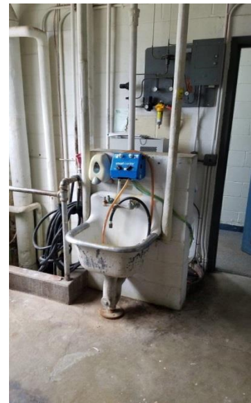
Mechanical/Plumbing Piping, Utility Sink
