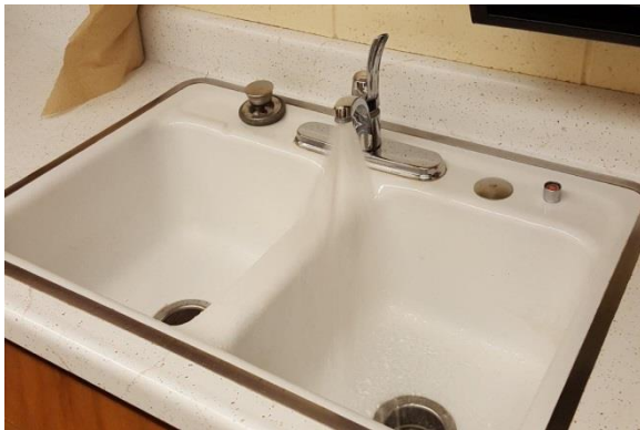
Faucet Working Incorrectly
