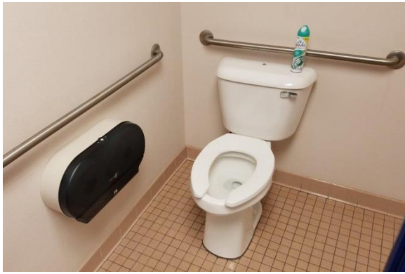
Missing Vertical Grab Bar at Men's Restroom
