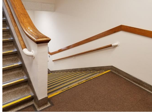
Missing Handrail Extensions at Stair S3
