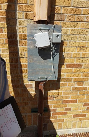
Abandoned Communication Wires
