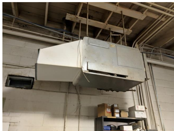
Abandoned Unit Heater
