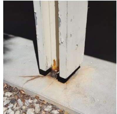
Rusted Column Post & Chipped Paint
