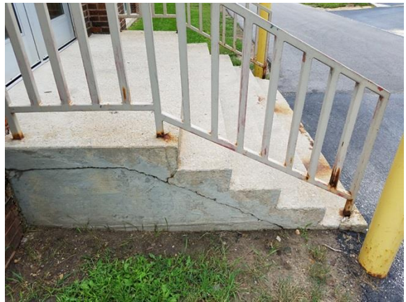
Rusting Railing Connections and Exposed/Rusting Steel
