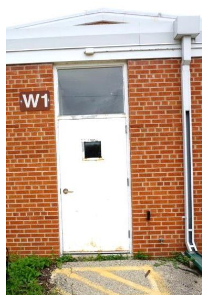
Rusted Door/Frame, Stoop Settlement at Exit/Entry
