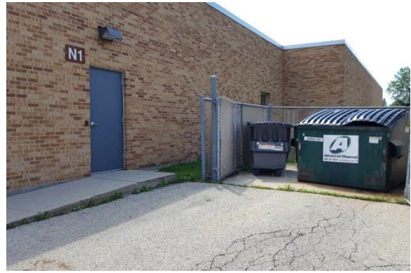
Ramp Not ADA Compliant; Deteriorated Dumpster Enclosure
