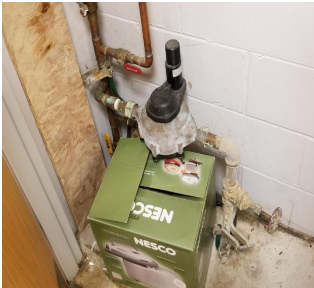
Water Service to Building
