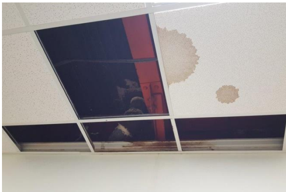
Ceiling Tile & Grid Stained & Missing Tiles at Corridor
