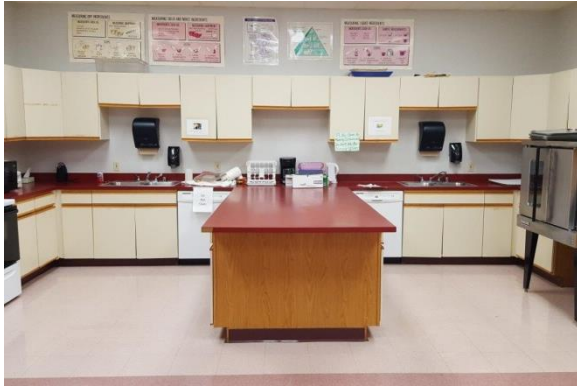
Sinks Don't Meet ADA Requirements
