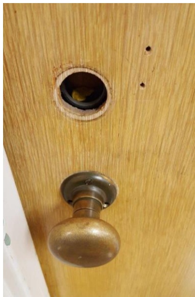
Missing Door Lock at Storage Door
