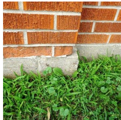
Spalling Masonry at Base of Wall
