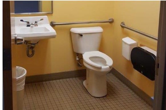
Missing Vertical Grab Bar at Women Restroom
