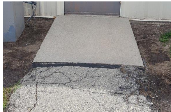
Unleveled & Cracked asphalt at Entry/Exit
