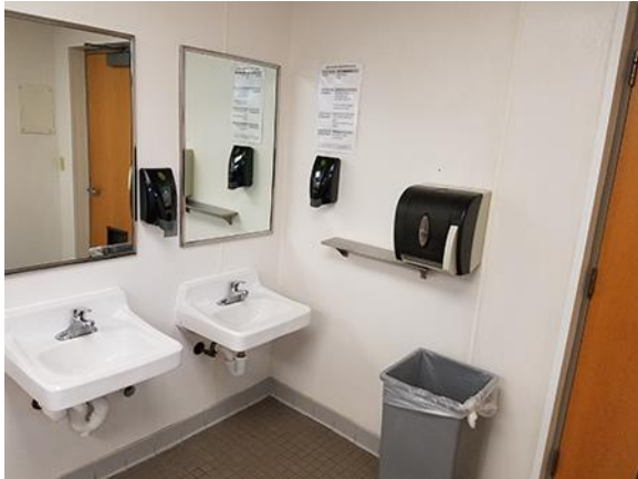
Mirror Not at ADA Compliant Height
