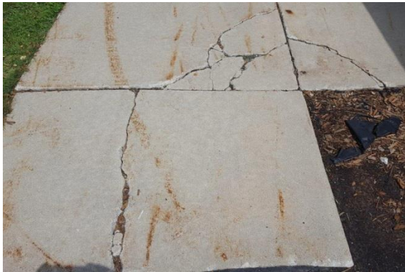
Cracks on Exterior Concrete Slab at Main Entrance
