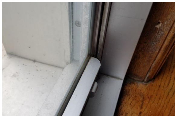
Single Pane Glazing at Original Building Classrooms
