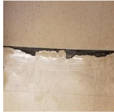
Damaged Vinyl Tile at Classroom 206
