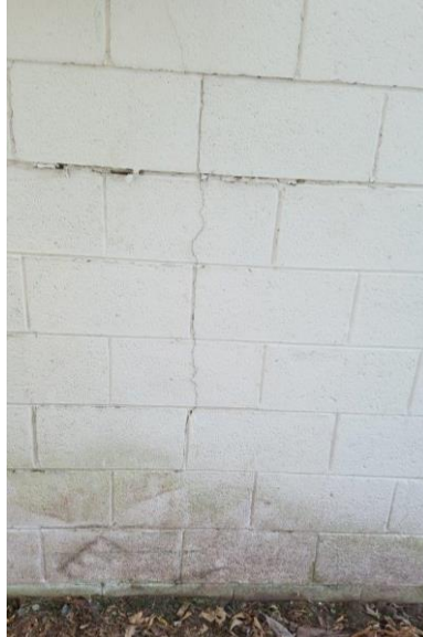
Foundation & Masonry Cracks
