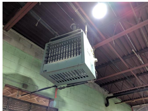
Empire Gas Fired Unit Heater
