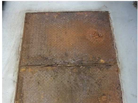
Rusted Floor Access Cover
