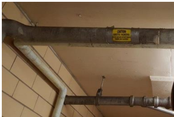
Asbestos on Mechanical Pipes
