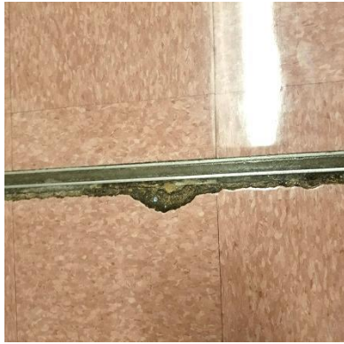
Chipping Vinyl Tile at Building Expansion Joint
