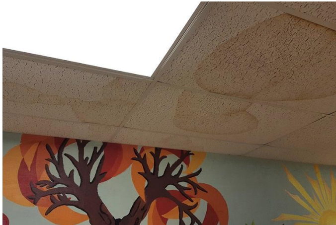
Water Damaged Ceiling Tiles
