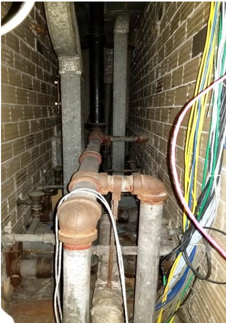
Plumbing Chase at Toilet Rooms
