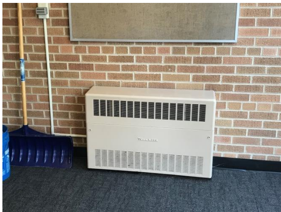
Cabinet Unit Heater
