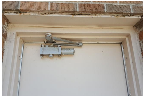
Rust at Steel Lintel
