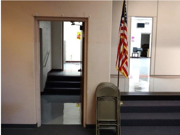
No ADA Access to Stage Area
