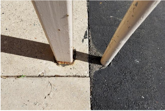
Rusted Column Base
