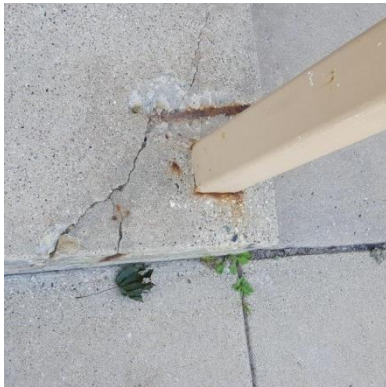
Rust at Exterior Column Base
