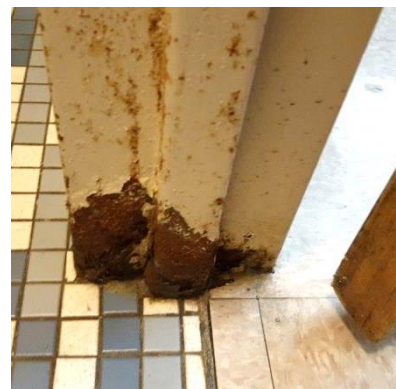
Rusted Door Frame Base at Kindergarten 112 - Bathroom
