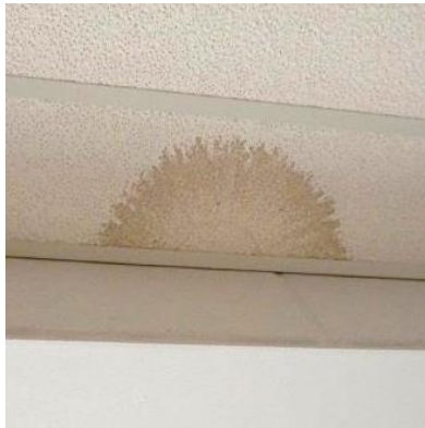
Stained Ceiling Tile at Multi-Purpose
