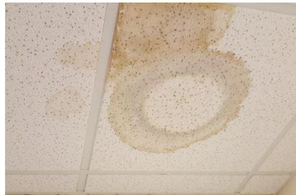
Ceiling Tile Stained by Water Damage at Workroom 231
