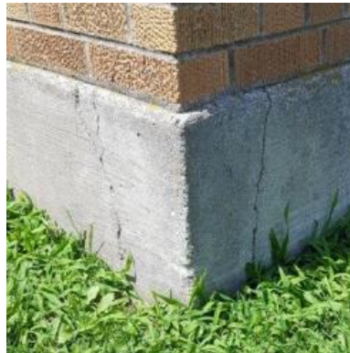
Foundation Crack at Corner
