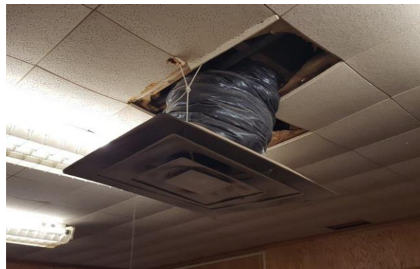
Deteriorated/Damaged Ceiling and Diffuser
