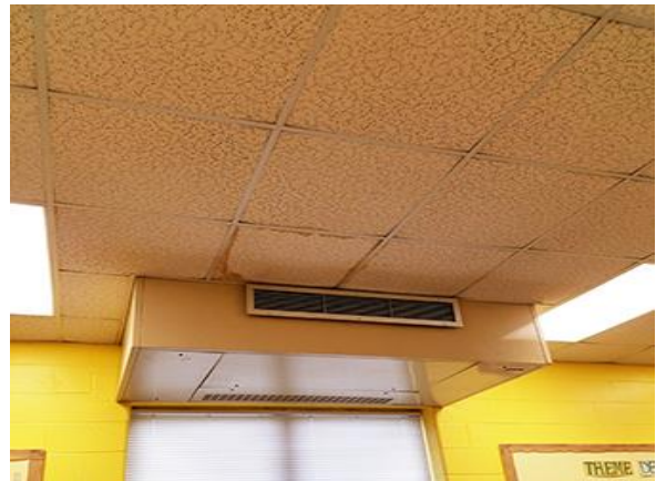
Ceiling Tile Degradation/Staining at Classroom 324
