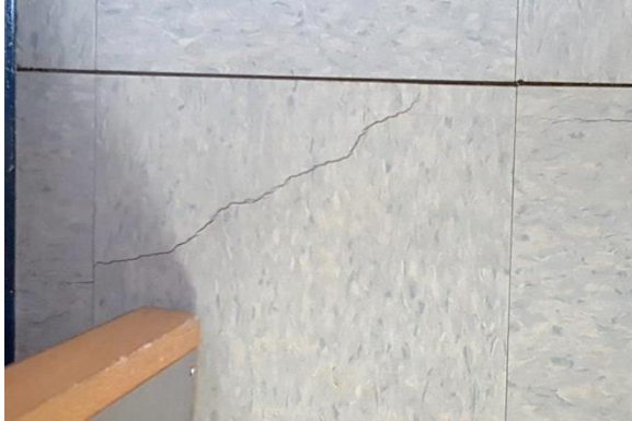
Cracked Vinyl Tile at Media Center - 207
