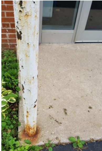
Rust at Canopy Column Base
