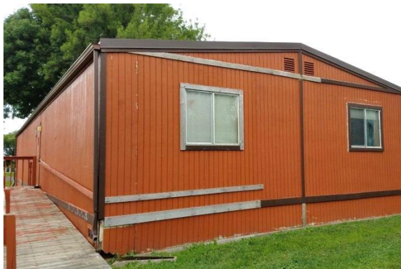
Exterior Envelope/Ramp Deterioration
