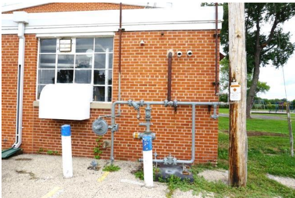
Piping/Ventilation at Mechanical Room Exterior
