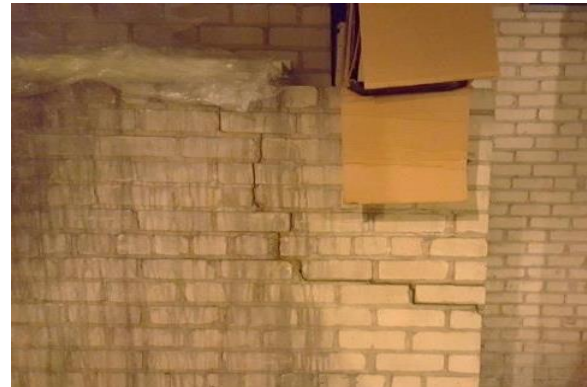
Cracks on Masonry Walls at Locker Room – Basement
