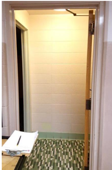
Non-ADA Compliant Toilet Vestibule Clearance at Boys Restroom
