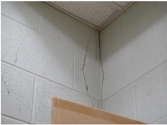
Structural Cracking at Masonry Wall Corner
