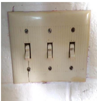
Broken Outlet Cover
