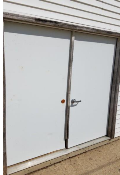
Doors in Deteriorated Wood Frame
