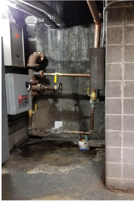
Water Service Piping
