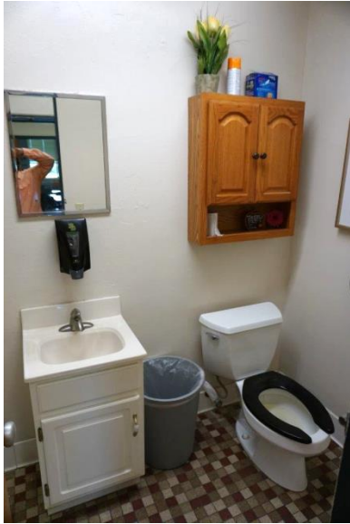
Non-ADA Compliant Staff Restroom
