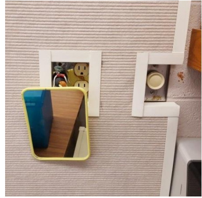
Electrical Components Concealed/ Enclosed at Classroom 116
