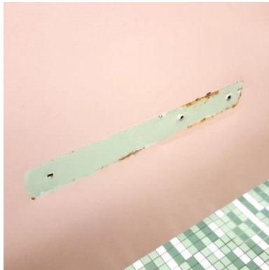
Missing Grab Bar at Girl's Restroom
