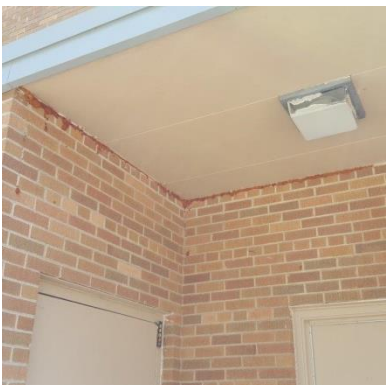
Exposed foam insulation at soffit
