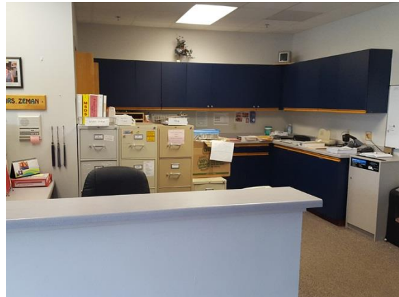
No ADA Transaction Counter at Reception
