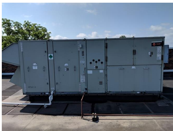
Trane Rooftop Unit
