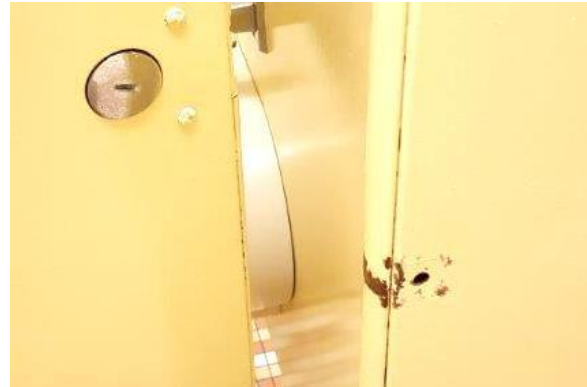
Missing/Damaged Privacy Locks on Toilet Partition Door at Staff Toilet Room
