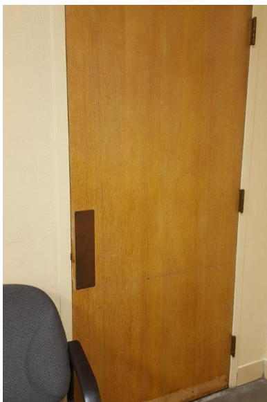
Abandoned Connecting Door at Staff Lounge 227
