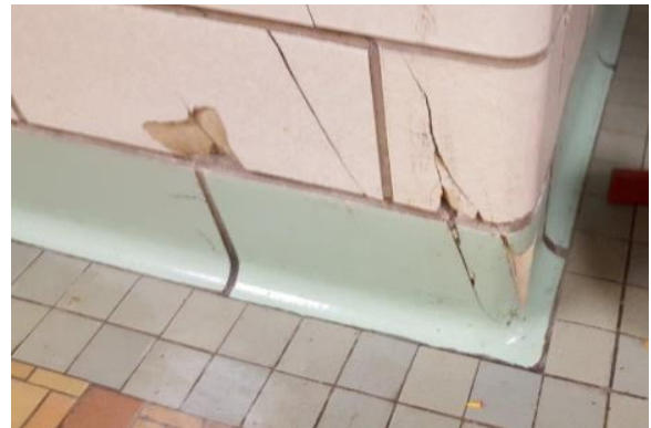
Damaged & Cracked Glazed CMU and Wall Base at Store Corridor
