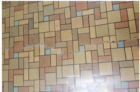
Cracks on Ceramic Tile Flooring
