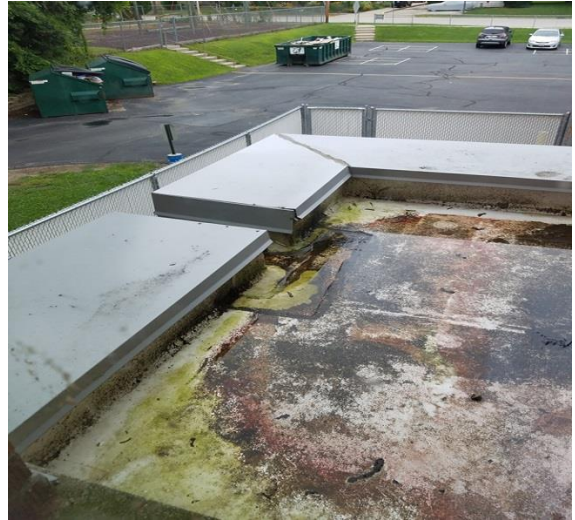
Standing Water/Algae Growth at Roof
