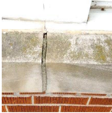
Concrete Lintel Deterioration
