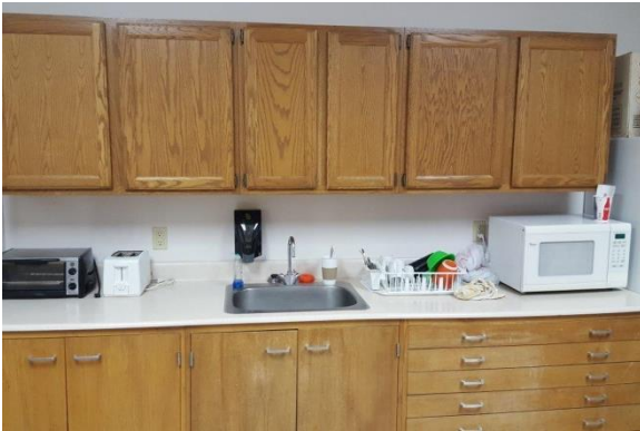
Non-ADA Compliant Counters/Fixtures at IMC Office Area
