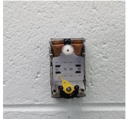
Missing Thermostat Cover
