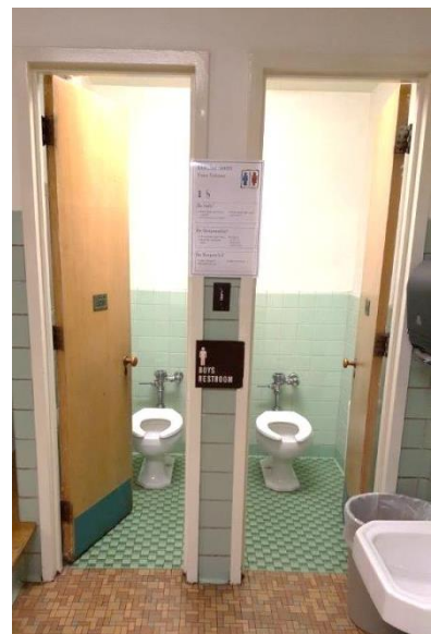
2 Shared Stalls Divided By Partition at Girl's Restroom – Not ADA
