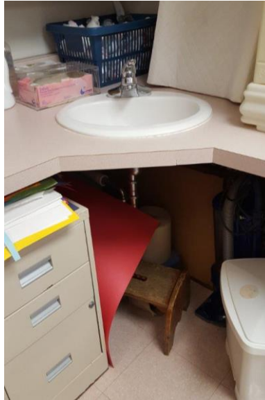
Sink Doesn't Meet ADA Requirements
