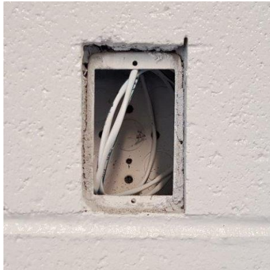
Missing Outlet Cover/Exposed Wires
