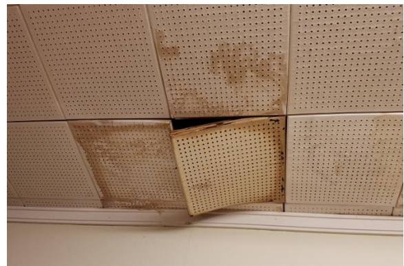
Ceiling Tile Deterioration and Staining at Classroom 302
