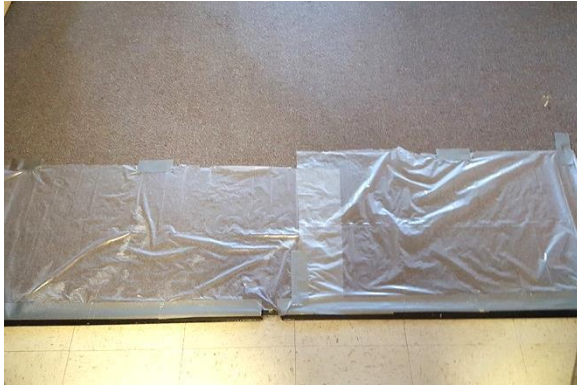
Damaged/Taped Carpet Transition at Classroom 100
