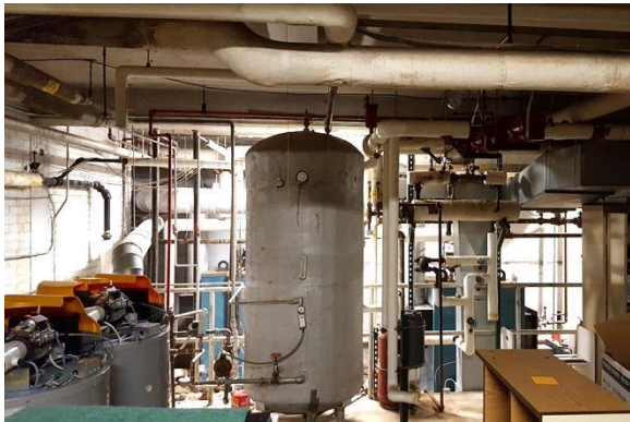
Boiler Room with Abandoned and New Equipment/Piping
