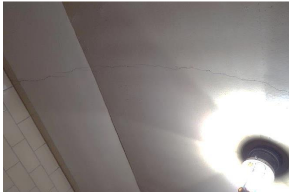
Cracks on Ceiling at Boiler Room – Basement
