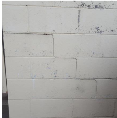
CMU Cracks & Peeling Paint
