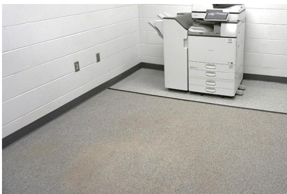
Heavy Carpet Staining at Copy Area
