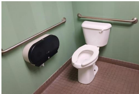
Missing Vertical Bar at Men Restroom 110
