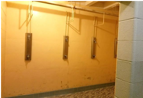
Abandoned Showers in Locker Rooms
