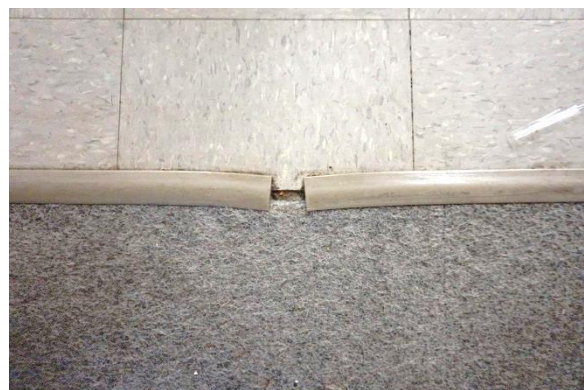
Missing Transition at Carpet/Vinyl Tile
