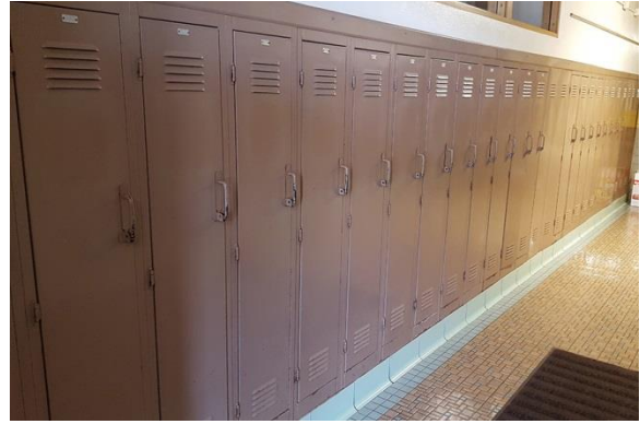
Rusting, Dented, and Scratched Metal Lockers
