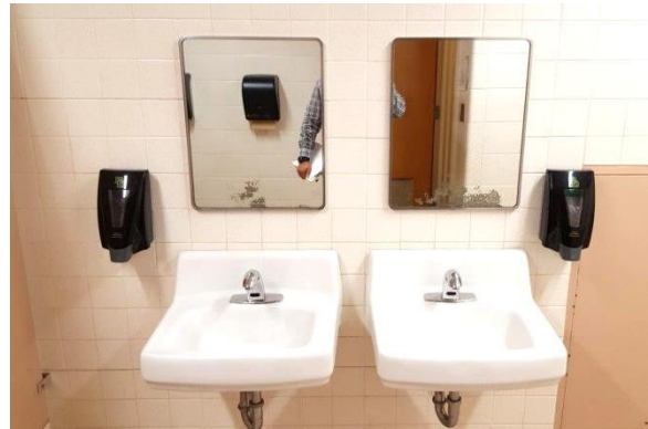
Non-ADA Compliant Sinks/Mirrors at Boy's Restroom
