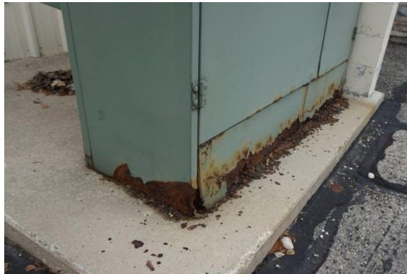
Major Rust on Base of Electrical Unit
