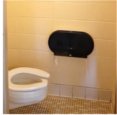
Missing Grab Bars at Kindergarten Restrooms
