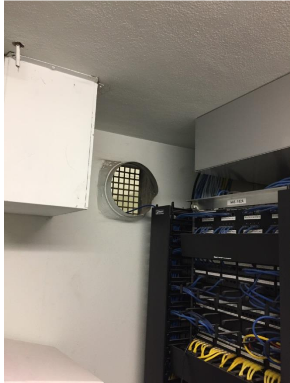
Transfer Duct to IT Area
