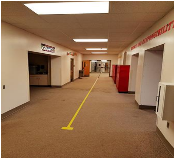
Heavy Staining at Corridor Carpet
