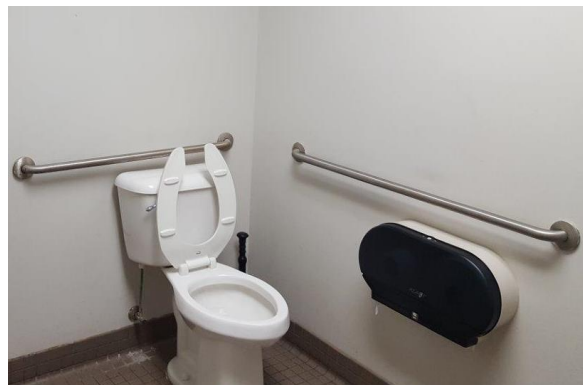
Missing Vertical Grab Bar at Women Restroom 109
