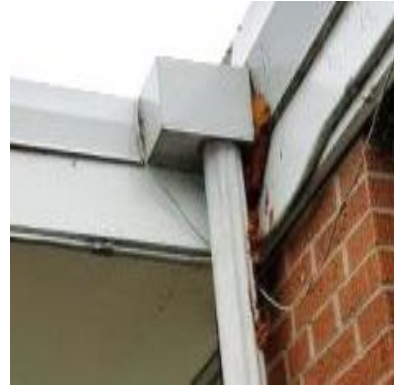
Leaking Conductor/Gutter; Exposed Insulation
