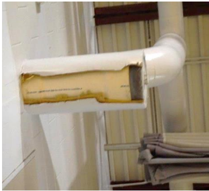
Damaged Insulation at Gymnasium
