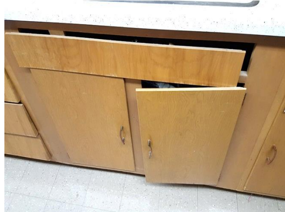
Damaged Wood Base Cabinet at Classroom
