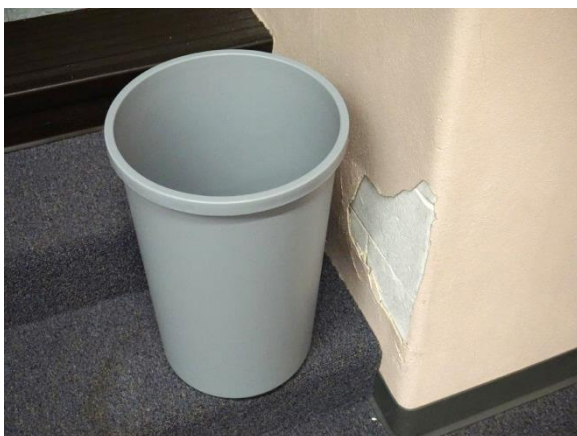
Missing Plaster at Base of Wall
