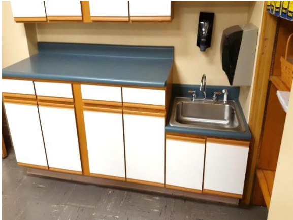
Non-ADA Compliant Casework/Sink
