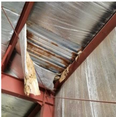
Deteriorated Metal Deck and Insulation
