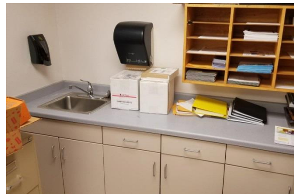
Non-ADA Compliant Counters/Fixtures at Break Room
