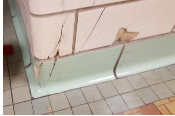
Damaged & Cracked Glazed CMU and Wall Base at Corridor
