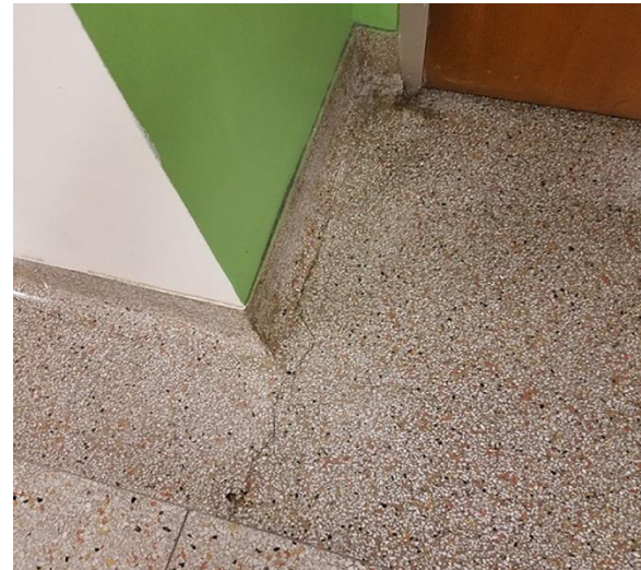
Cracked Terrazzo at Room Entry
