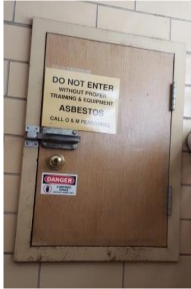
Asbestos Notification at Chase
