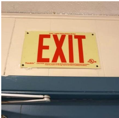
Non-Illuminated Exit Sign
