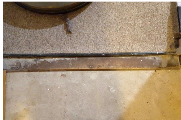
Damaged Floor Transition at Gym – Storage Room
