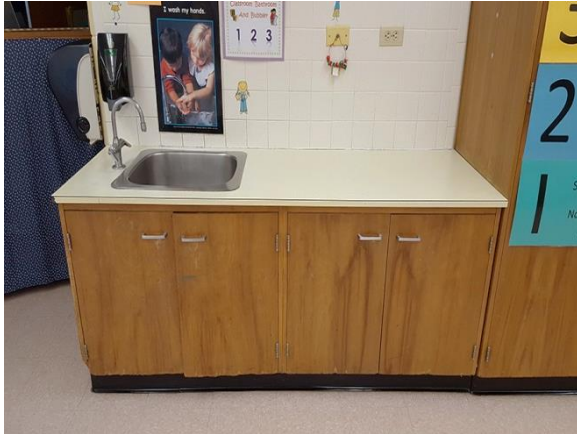
Non-ADA Compliant and Damaged Casework/Sink at Classroom
