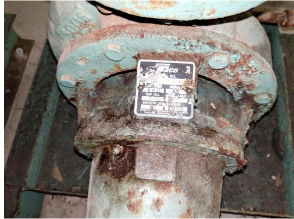
Base Mounted Taco Pump
