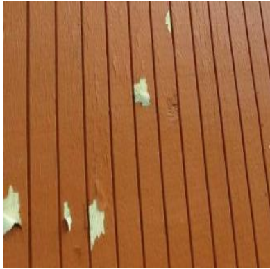
Flaking Paint at Wood Cladding
