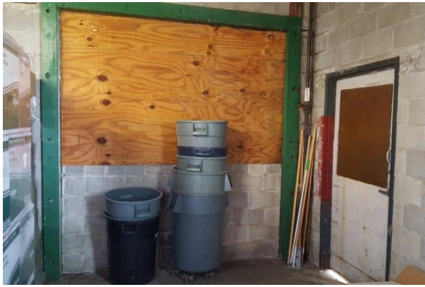
Boarded Up Garage Opening & Door Window
