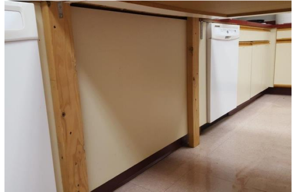
2x Wood Support to Island Countertop
