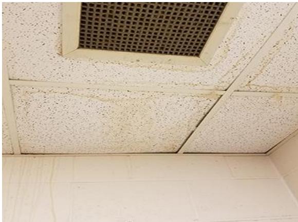
Ceiling Tile Staining at Storage Room
