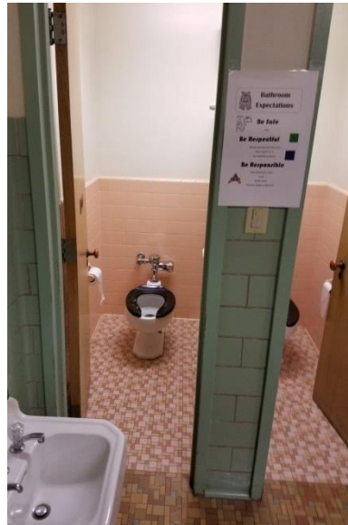
2 Shared Stalls Divided By Partition at Girl's Restroom
