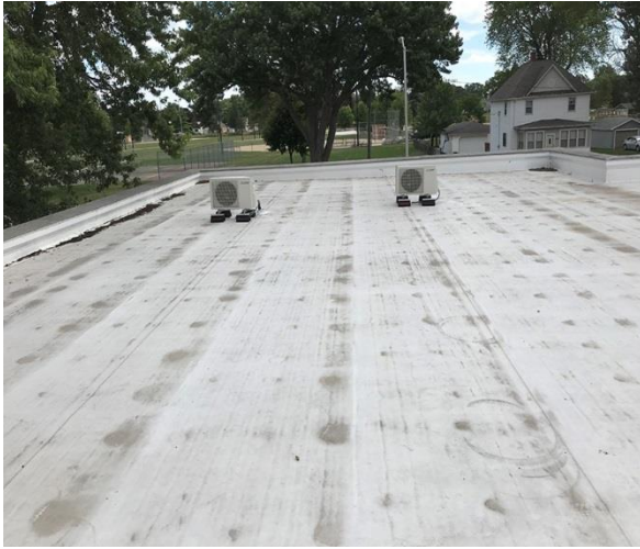
TPO Roofing with Scrim Showing
