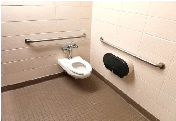
No Vertical Grab Bar Installed at ADA Toilet Stall
