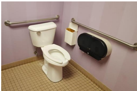
Missing Vertical Grab Bar at Men Restroom
