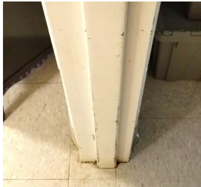
Scratched/Rusted Door Frame
