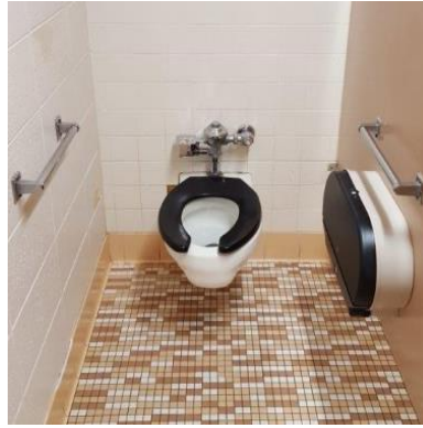
Incorrect/Missing Grab Bar Locations; Clearance Issues at Boy's Restroom
