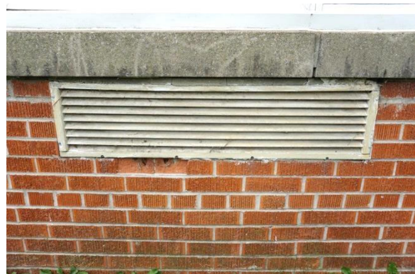
Rusted and Damaged Louver
