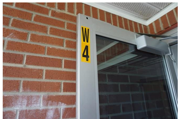
Efflorescence on Brick at Entry W4
