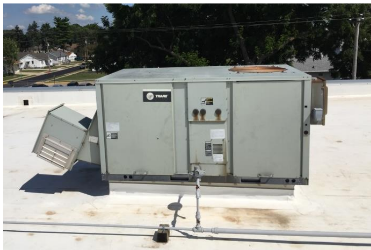
Trane Roof Top Unit
