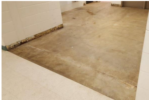
Missing Flooring & Baseboard at Corridor
