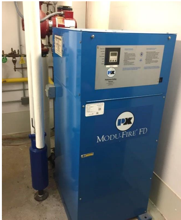
Patterson Kelley Condensing Boiler
