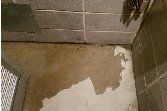
Water Leakage at Boiler Room
