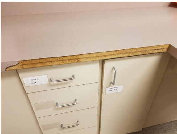
Damaged Plam Counter at Room 206
