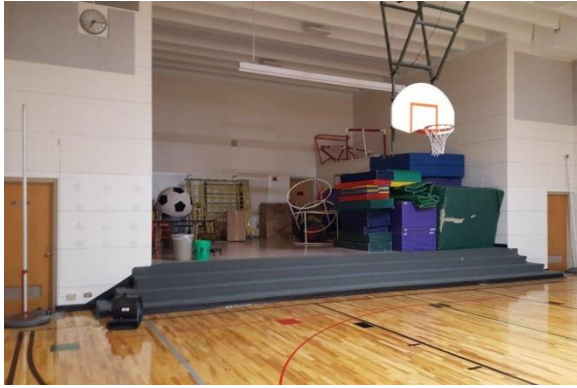
No ADA Ramp Access to Stage Area
