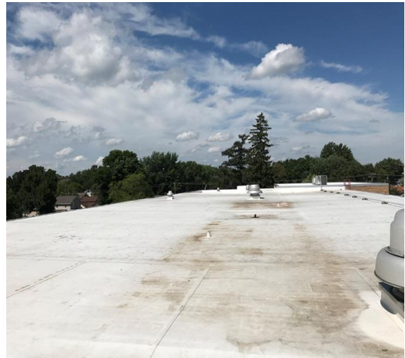
Roof Scrim Showing Through Membrane
