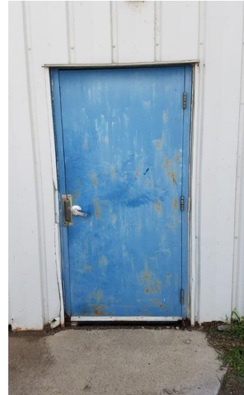
Damaged Exterior Door
