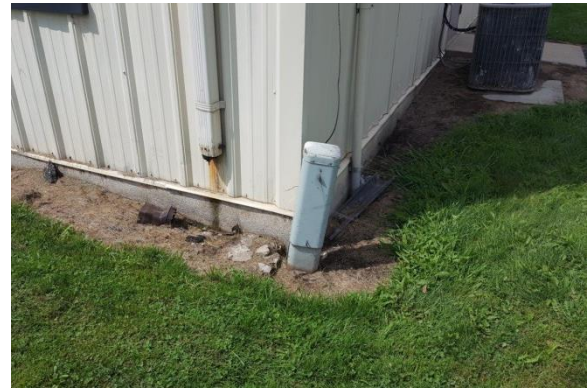
Displaced Electrical Equipment, Missing Downspout
