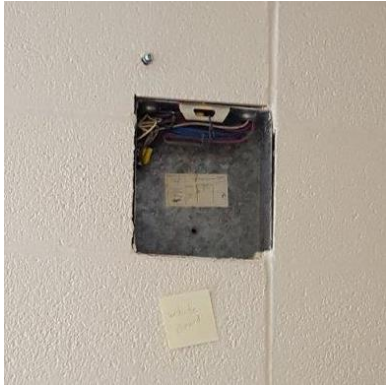
Exposed Wiring & Missing Covers at Classrooms
