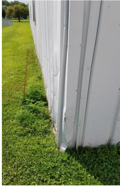
Damaged Metal Siding Corner
