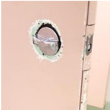
Broken Privacy Lock at Girl's Restroom
