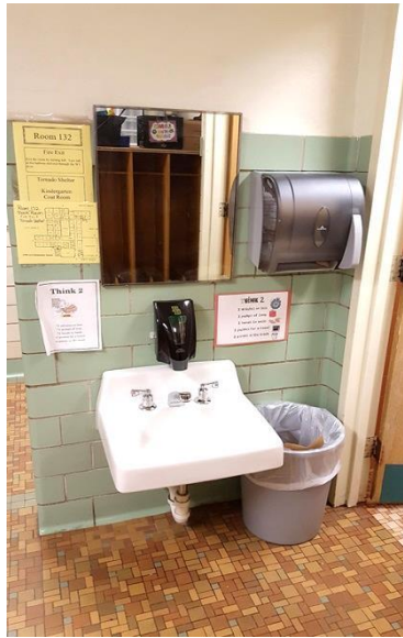
Non-ADA Compliant Plumbing Fixtures
