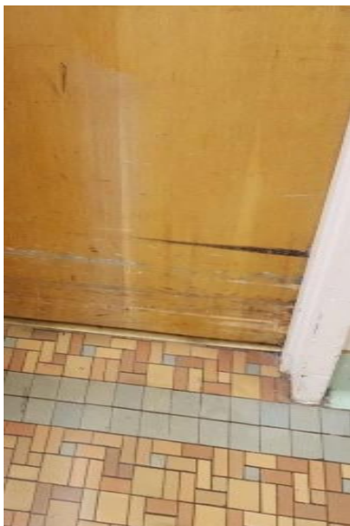
Missing Door Plate & Damage
