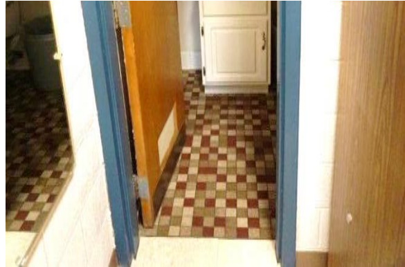
Non-ADA Compliant Door (24") at Staff Restroom
