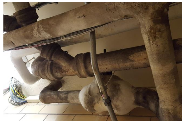
Asbestos on Plumbing Pipes
