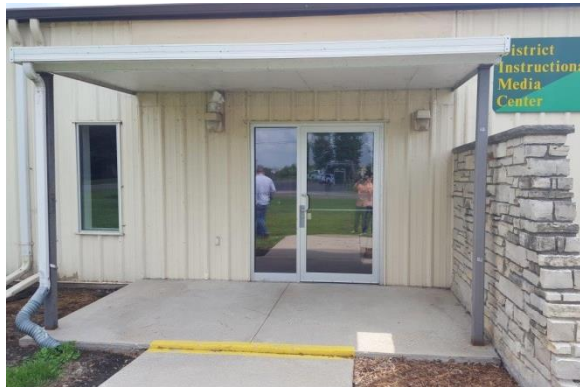
Non-ADA Compliant Entry, Rusted Column Base at S-2 Entrance – Pupil Services
