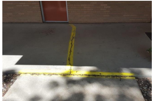
Cracks on Exterior Concrete Slab at Sidewalk
