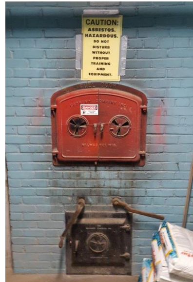
Asbestos Notification at Boiler Room
