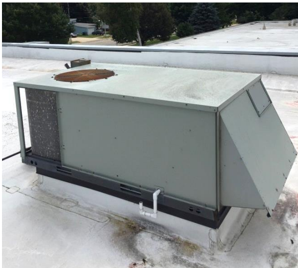
Trane Rooftop Unit
