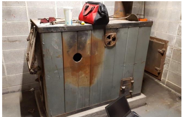
Abandoned Mechanical Equipment
