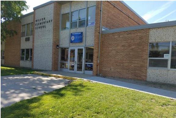
Non-ADA Compliant Main Entry
