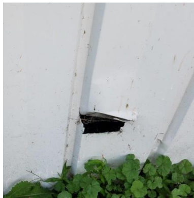
Damaged Metal Siding
