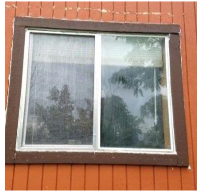
Deteriorated Single Pane Window
