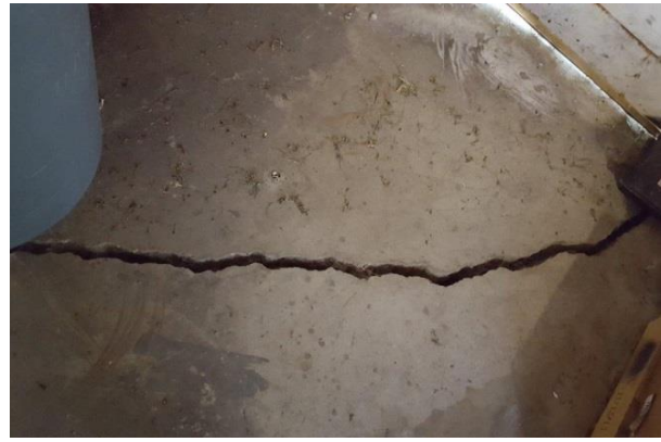
Concrete Slab Cracks
