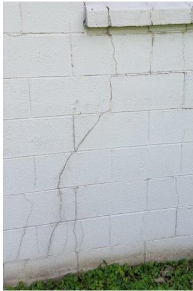
Cracking From Window Opening to Foundation
