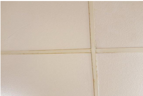
Ceiling Grid Rusting at Women's Restroom
