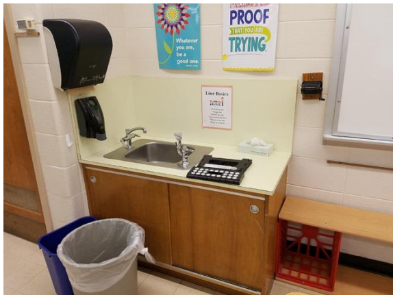
Non-ADA Compliant Casework/Sink at Class Rooms
