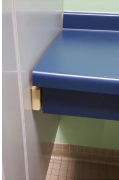
Wood Shim Support for Sink Counter at Men Restroom 110
