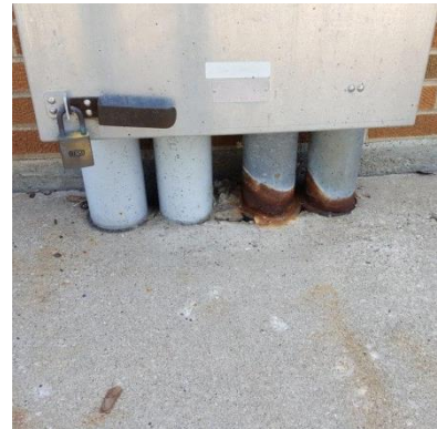
Rusting at Electrical Equipment
