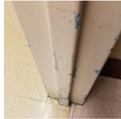
Scratched Door Frame
