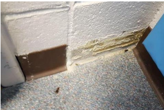
Missing Wall Base Transition
