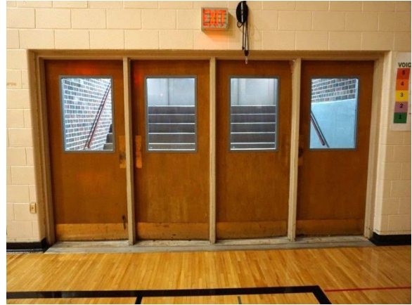
Missing Panic Hardware at Exit Doors
