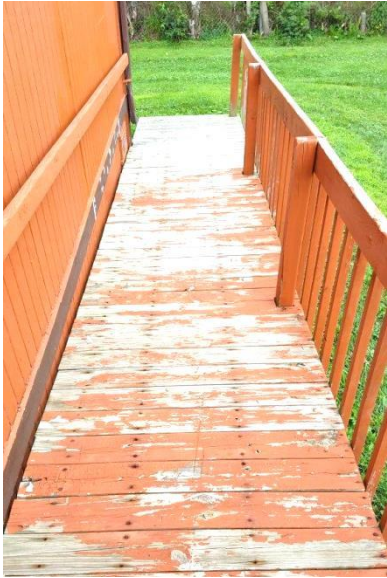
Non-ADA Compliant Ramp, Structure Deteriorating
