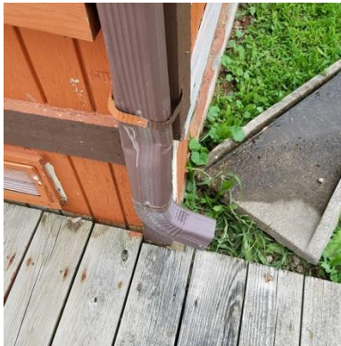
Improper Drainage; Rotted Wood Decking
