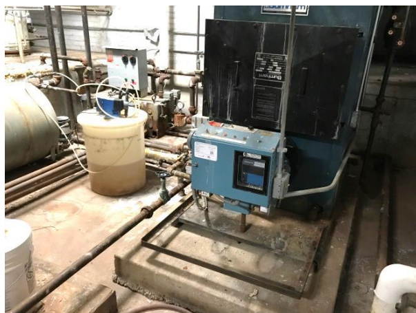
Burnham Fire Tube Boiler
