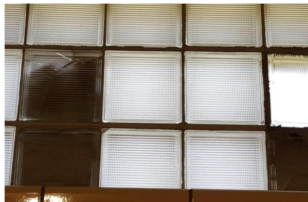
Cracked Glass Block Windows at Basement Locker Rooms
