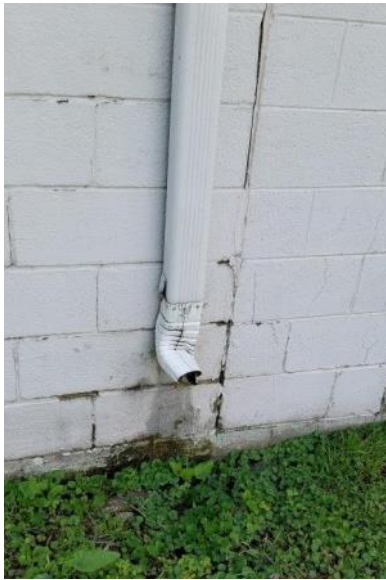
No Downspout Termination
