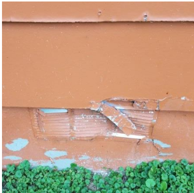
Dented & Damaged Vent & Siding
