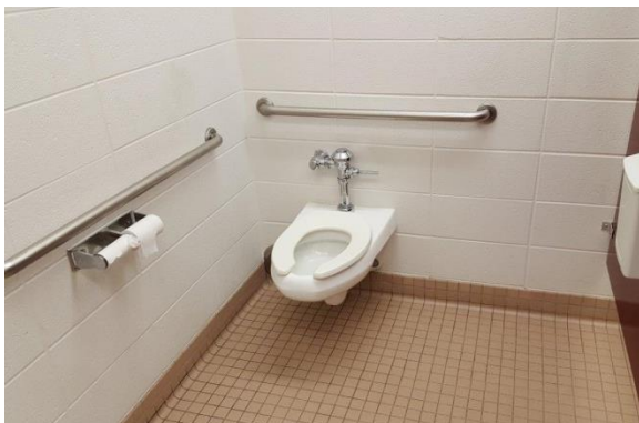
Missing Vertical Grab Bar at Men's Restroom
