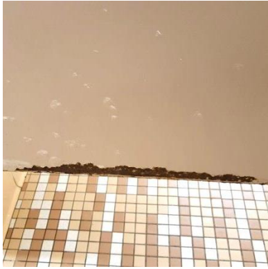
Rust on Toilet Partition
