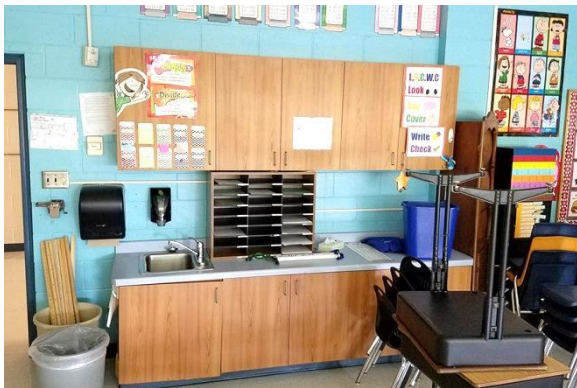
Non ADA Compliant Casework at Classroom 102
