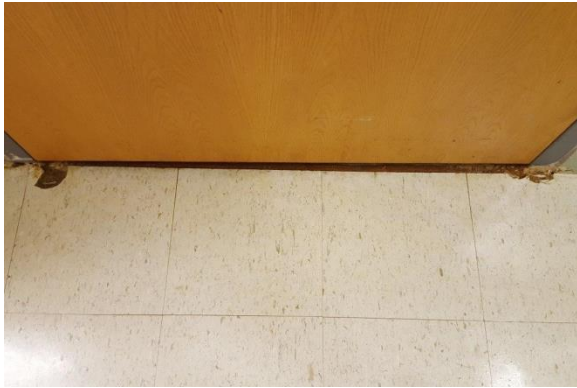
Broken Tile at Corridor Storage Door
