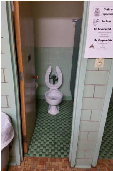
24" Door at Women Restroom – Office
