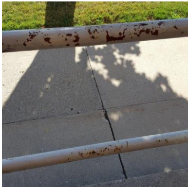
Rust at Handrails
