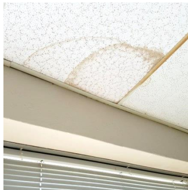
Ceiling Tile Grid Sagging & Stained at Kindergarten Room 112
