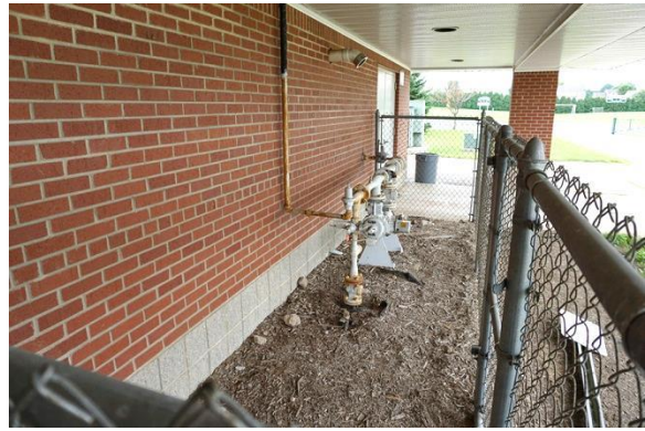
Rusted Pipes Between Entrances W-4 & W-3
