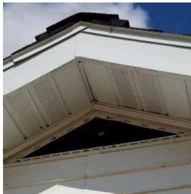
Missing Vinyl Siding
