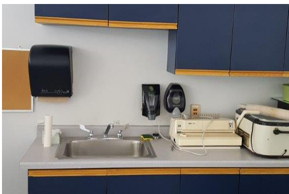
Sink Doesn't Meet ADA Requirements
