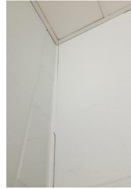
Cracked CMU Wall
