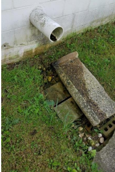
Erosion of grade at Roof Conductor Outlet
