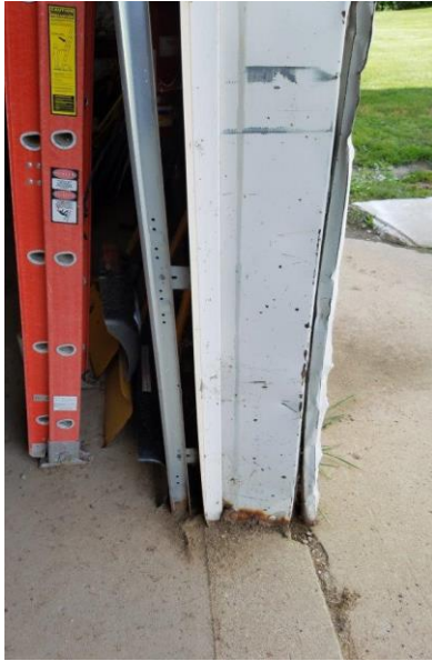
Damaged Overhead Door Jamb
