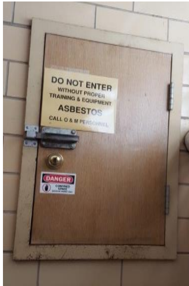
Asbestos Notification at Chase
