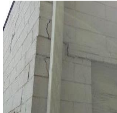
Major Cracking/Displacement at CMU Corner
