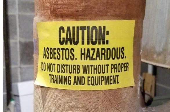
Asbestos Contamination Indicated at Boiler Room
