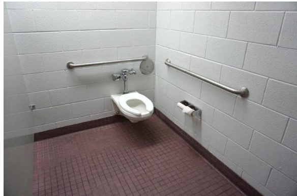
Missing Vertical Bar at Women's Restroom
