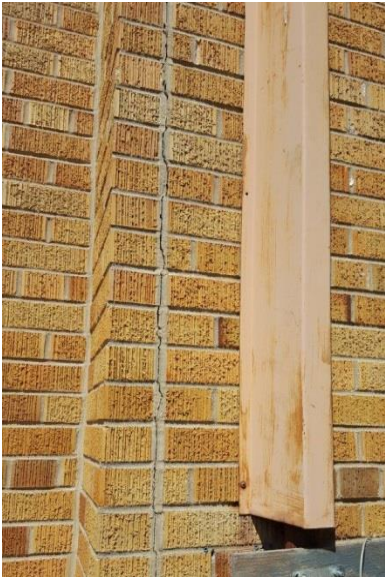
Masonry Control Joint Cracks
