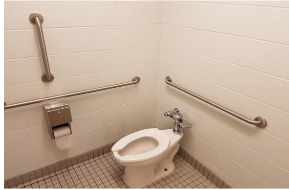
Vertical Grab Bar Installed at Child Restroom
