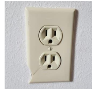
Damaged Outlet Cover
