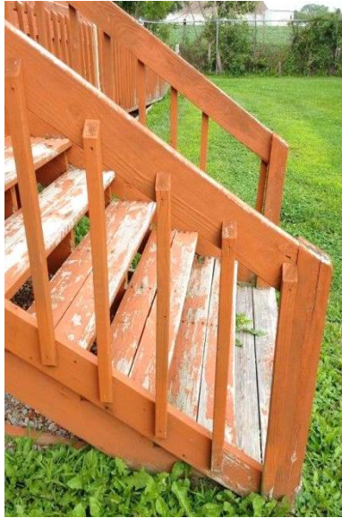
Non-Code Compliant Wood Stair Deteriorating, Paint Flaking Off
