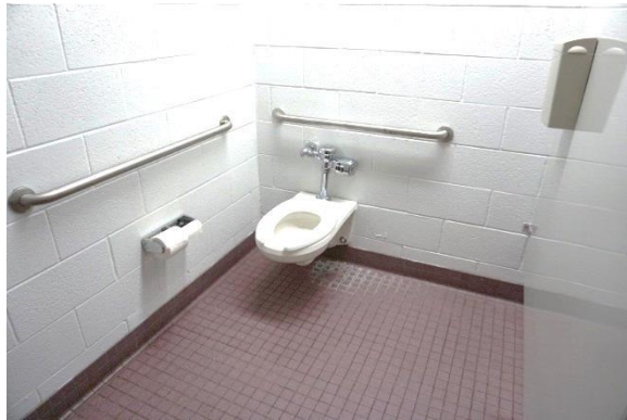
Missing Grab Bar at Men's Restroom
