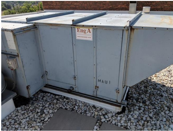
Engineered Air Make-up Air Unit
