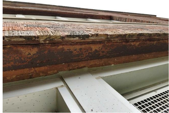
Rusted Lintel, Deteriorated Caulk/Flashing
