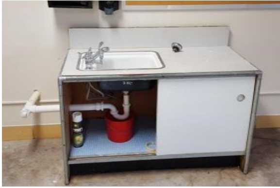
Exposed Plumbing, Damaged Millwork at Classroom 302
