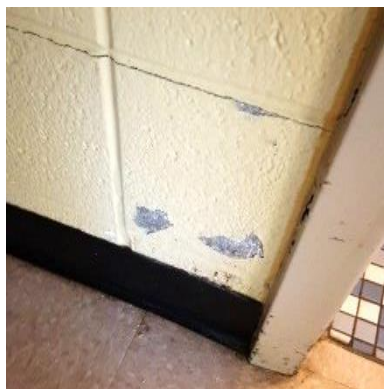
CMU Wall Cracks & Chipping Paint at Kindergarten 112 - Bathroom
