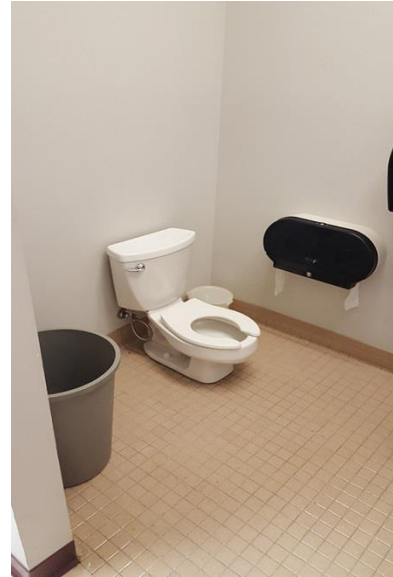
Missing Grab Bars at Child Restroom
