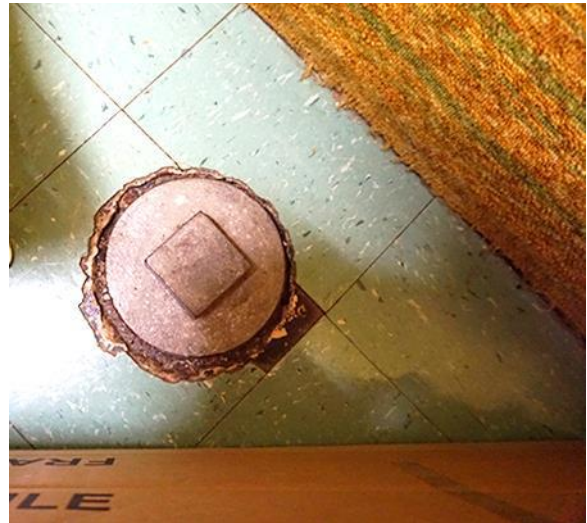
Vinyl Tile Deterioration at Penetration in Music Room
