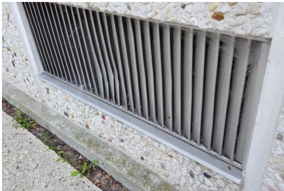
Damaged & Dented Louvers
