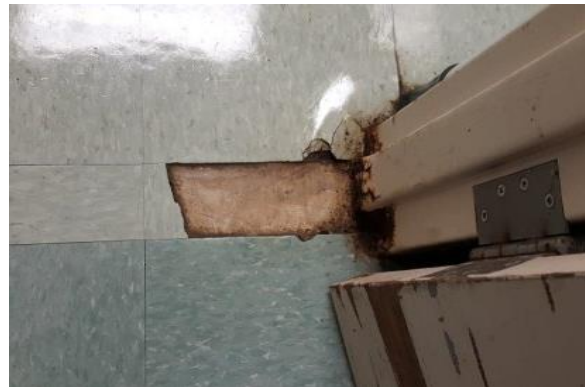
Damaged Vinyl Tile and Rusted Metal Door Frame
