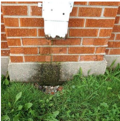
Missing Downspout, Foundation Discoloration
