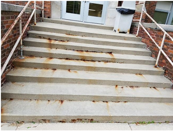
Deteriorated Exterior Stairs and Railings
