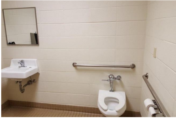
Lack of Vertical Bar at ADA Restroom
