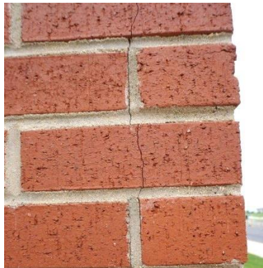
Cracks on Brick Façade
