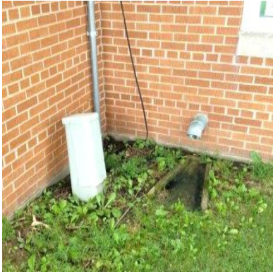
Improper Conductor Termination, Grade Settlement
