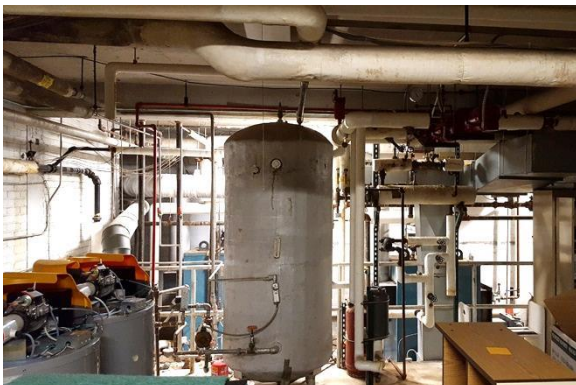
Boiler Room with Abandoned and New Equipment/Piping
