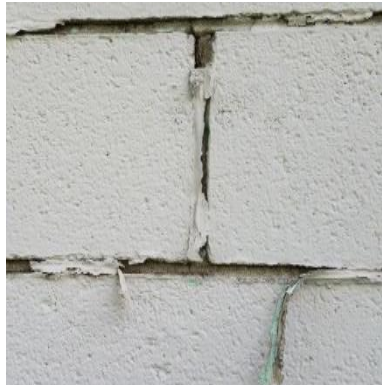
Failing Mortar Joints
