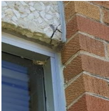
Cracked Masonry at Window Edge
