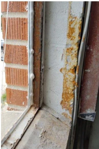
Rusted Window Frame/Deteriorating Caulk
