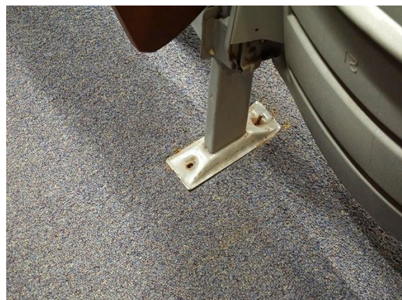
Missing Hardware at Auditorium Seats
