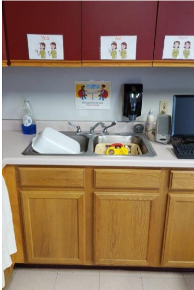
Sink Doesn't Meet ADA Requirements
