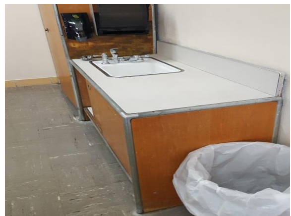
Damaged Non-ADA Compliant Casework at Classroom
