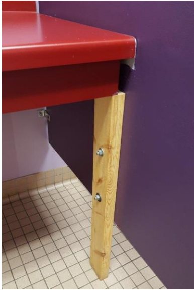
Wood 2x Framing Bolted to Partition at Women Restroom 109
