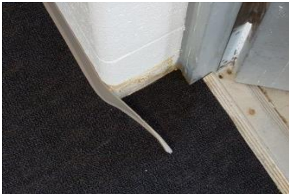
Lifting Wall Base at E2 Main Entrance
