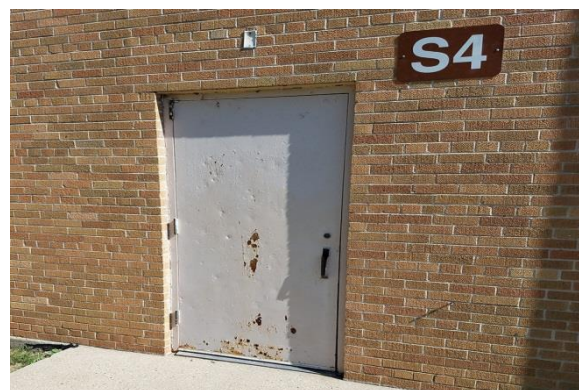
Rusted Exterior Door at Exit S4 handrails
