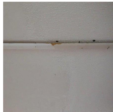
Ceiling Water Damage at Staff Restroom
