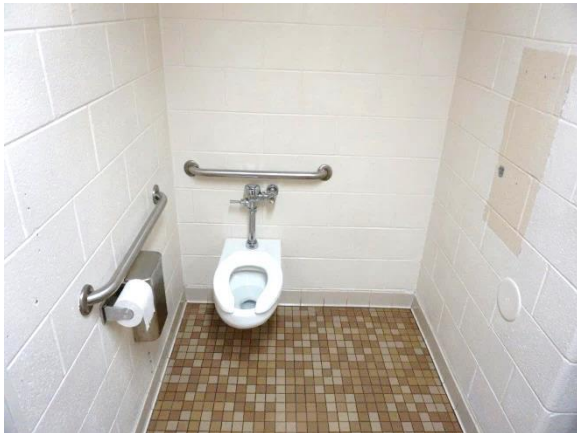
Missing Vertical Grab Bar
