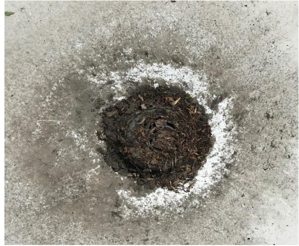
Deteriorated/Plugged Roof Drain
