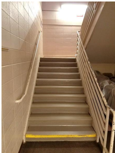
Chipped Paint at Railing and Stair Tread
