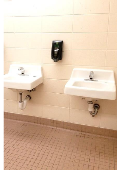
Non-ADA Compliant Lavatory
