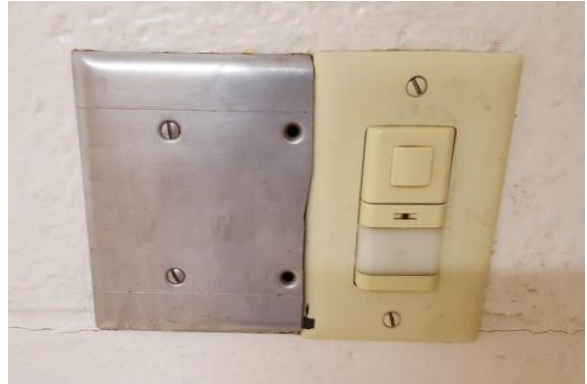
Custom-made Switch Cover at Boy's Restroom
