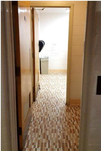
Non-ADA Compliant Toilet Vestibule Clearance at Girls Restroom
