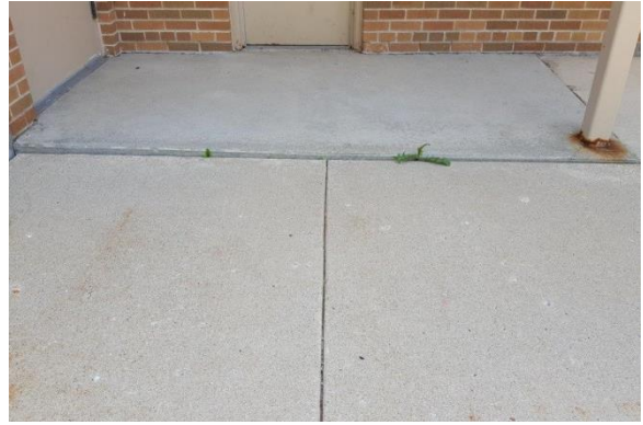
Heaving/Displaced Walk/Stoop at Exit
