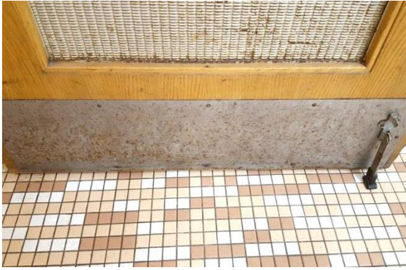
Rust on Door Plate at Boys & Girls Bathroom
