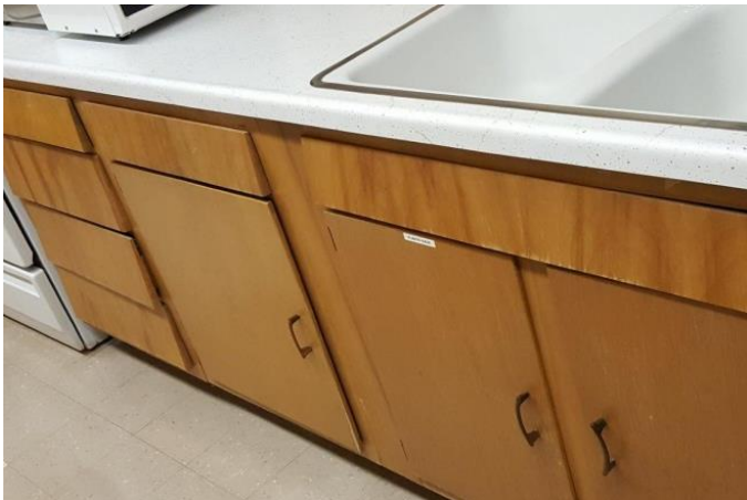
Old and Worn Non-ADA Compliant Casework
