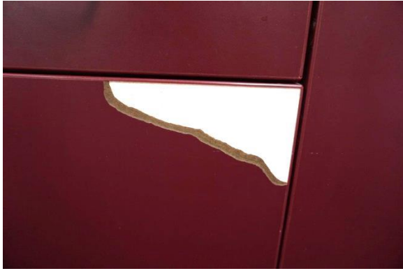
PLam Chipping on Casework
