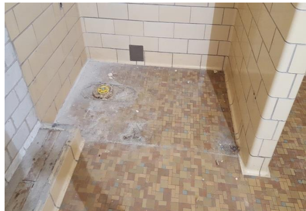
Abandoned Plumbing Fixtures at Locker Room
