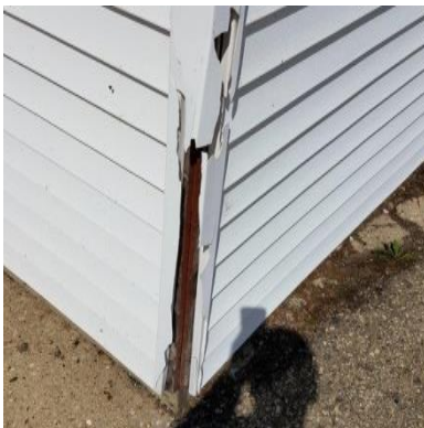
Cracked Vinyl Trim
