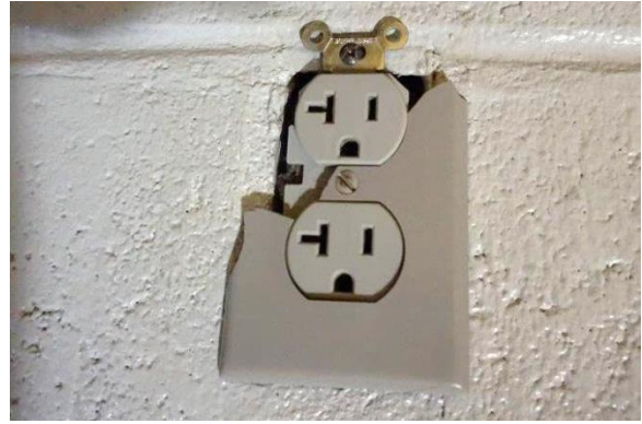
Broken Outlet Cover
