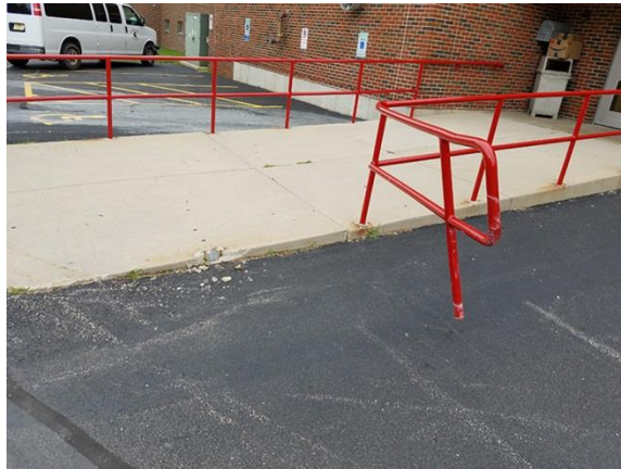
Damaged Exterior Railing
